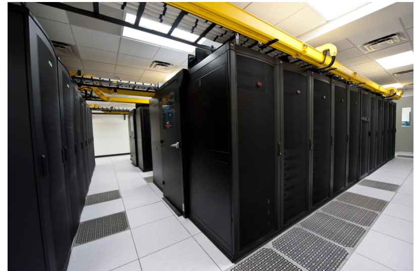
NREL Data Center storage arrays
