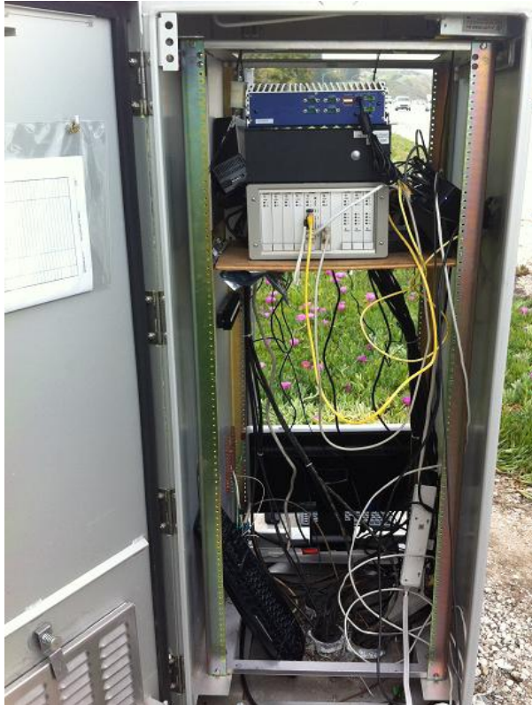
SR-57 SB Orange Station iSinc Controller running at diagnosis mode
