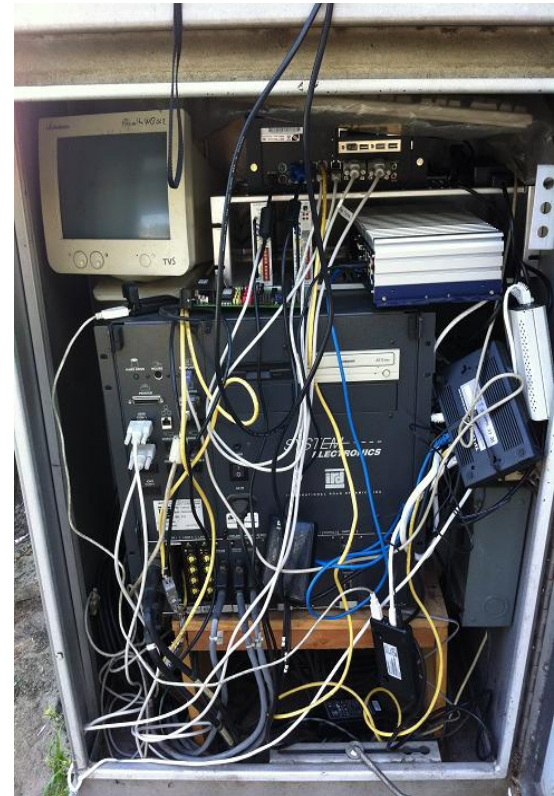
I-5 SB Irvine Station 1060 series controller with a customized solution from UCI
