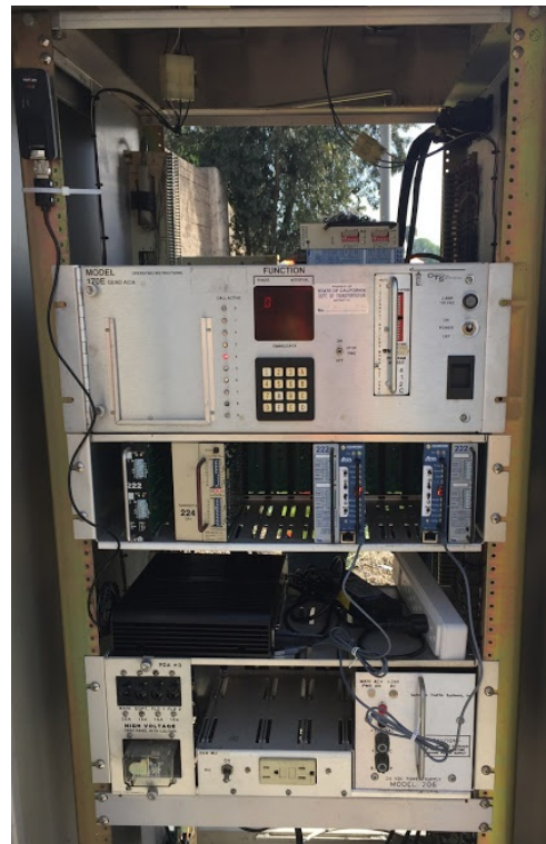
Ramp Metering ILD Site on SR-91 in LA
