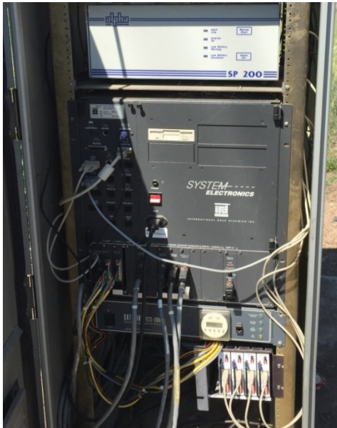
WIM Site on SR-99 between Stockton and Sacramento
