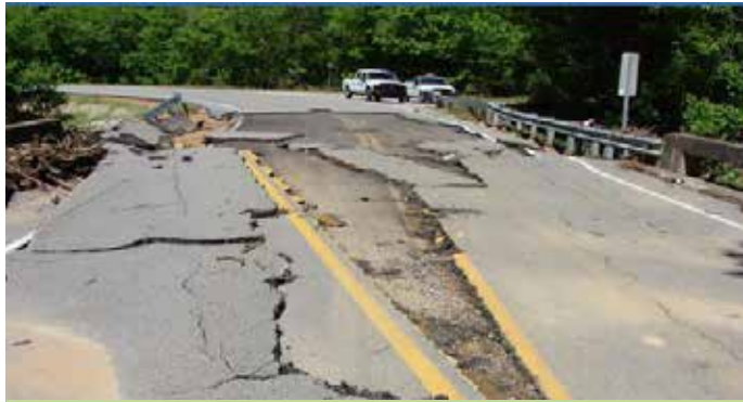
Approach Roadway Damage
