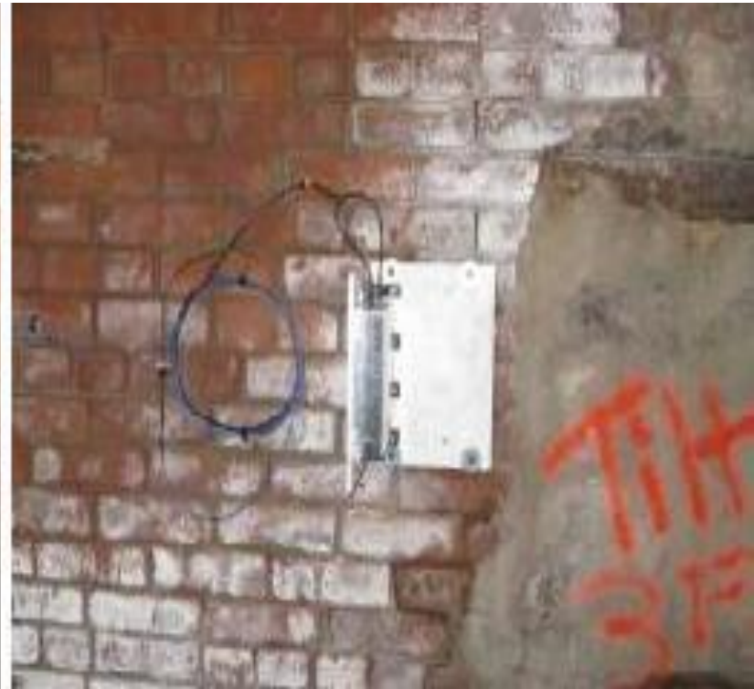
Typical FBG Tilt meter (wall supporting the two vaults)
