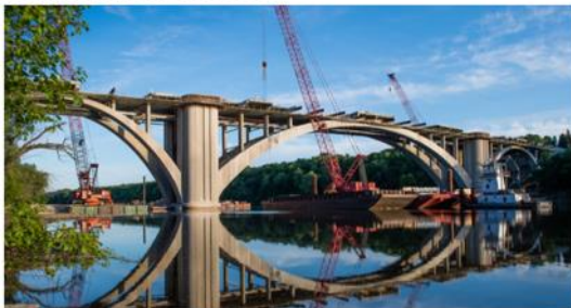
The Franklin Avenue Bridge is a historic crossing in downtown Minneapolis, MN, heavily used by drivers, pedestrians, and cyclists. Hennepin County used UHPC connections between precast deck panels to help accelerate the bridge's rehabilitation in 2016.
