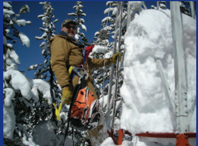
Although it sometimes requires tall climbs in mountain weather, regular maintenance of Montana's unique, historic network of lighted airway beacons is more cost-effective than taking the beacons down.
