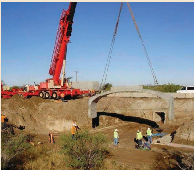
Figure 2. One of fifteen pre-cast concrete arches is dropped into place during the construction of one of two wildlife underpasses along State Route 86 in the Kitt Peak Wildlife Linkage in southwest Arizona. Note the small box culvert that the wildlife underpass replaced. Photo courtesy Arizona Department of Transportation.
