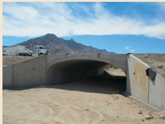
Figure 3. The finished eastern-most wildlife underpass on State Route 86 on the Tohono O’odham Nation in southwest Arizona. Photo courtesy Coalition for Sonoran Desert Protection.
