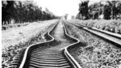
Fig. 1 – Buckling of Rails ( http://nisee.berkeley.edu )
