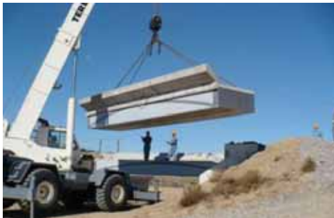
One of eight 30-foot hybrid composite bridge beams is installed for load tests in a railroad test track.
