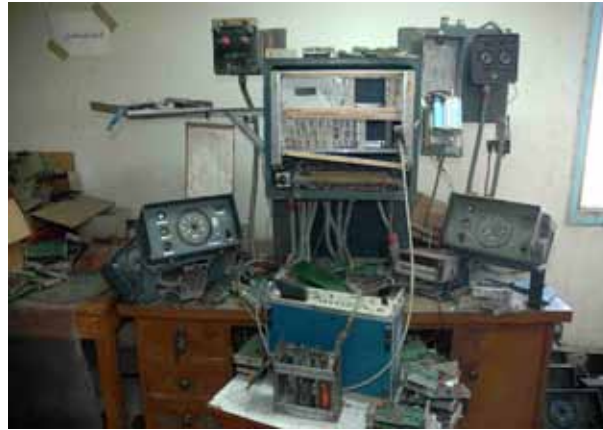
ATP test and repair facility. This desk is typical of many others.
