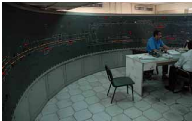
Centralized train control for trains into and out of Ramses Station, Cairo.
