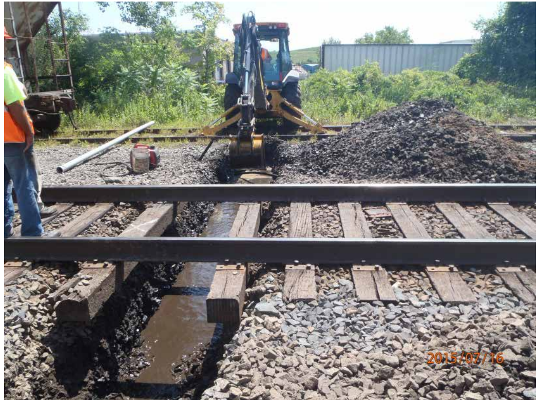
Cross-track excavation at MIDLAND Interlocking in Hartford, Connecticut. (Photo: NHHS Rail Program)
