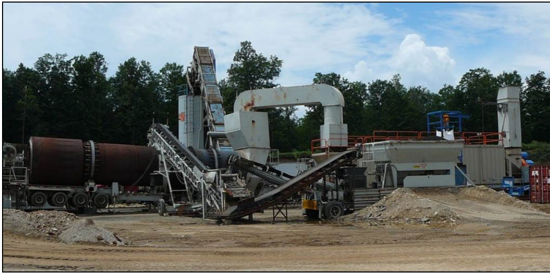
Figure 64 Parallel Flow Portable Drum Plant in Rapid River, MI
