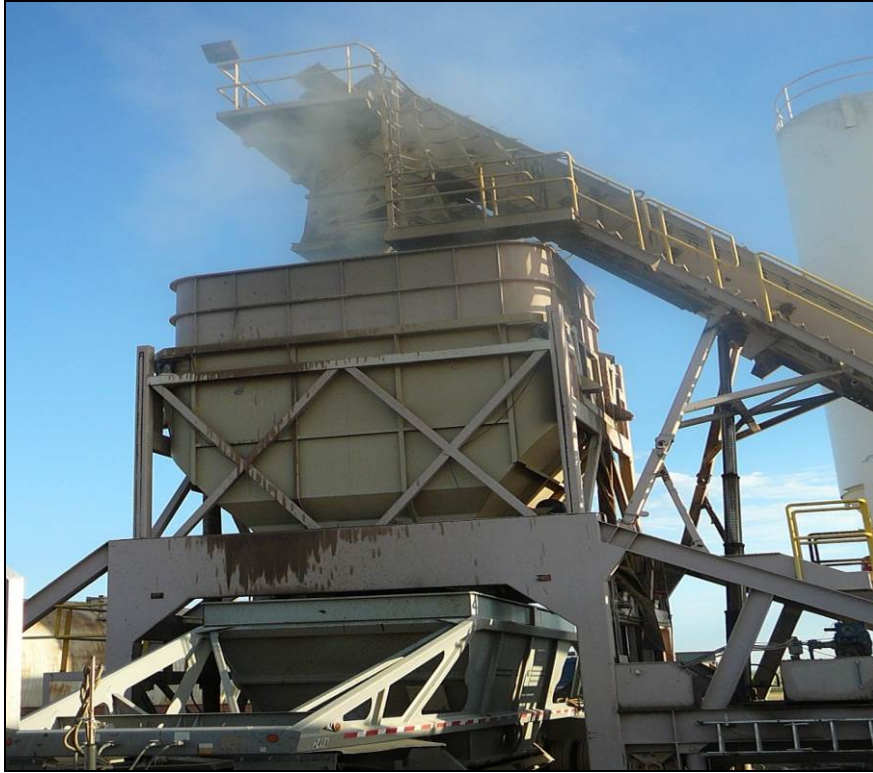
Figure 74 Portable Parallel Flow Drum Plant in Baker, MT
