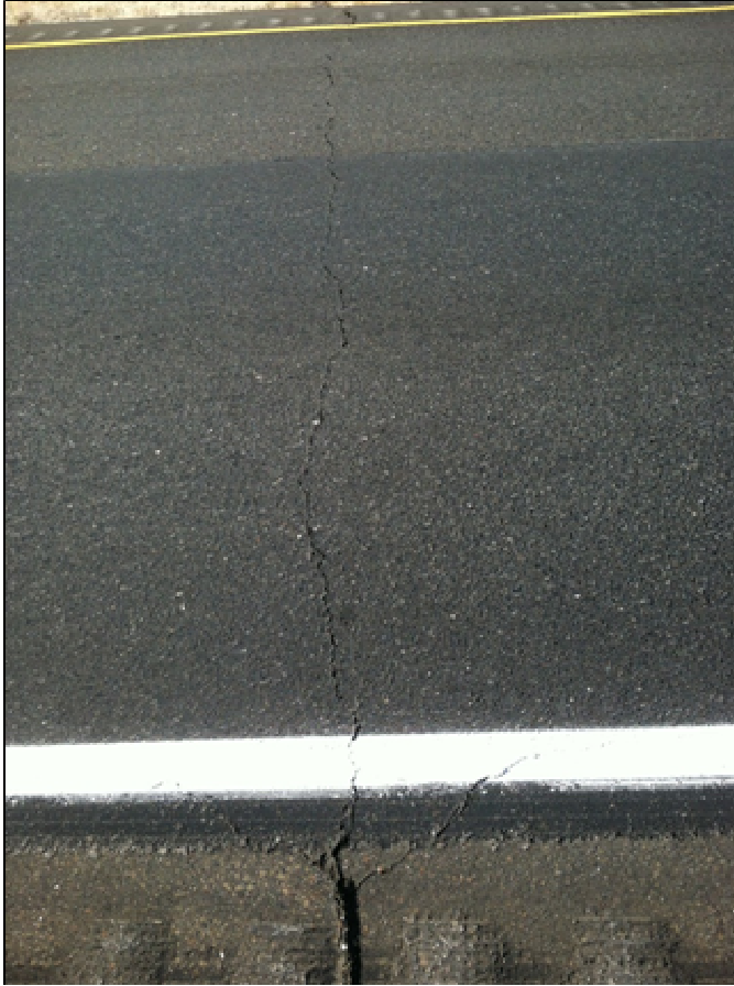
Figure 38 Example of Transverse Cracking in George, WA
