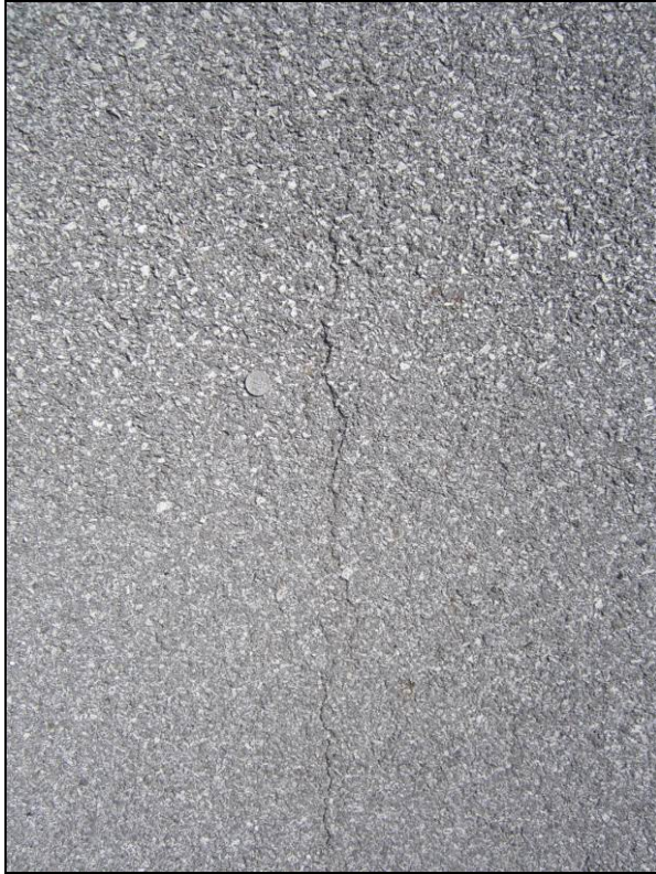
Figure 87 Example of Low-Severity Non-Wheelpath Longitudinal Crack in Munster, IN
