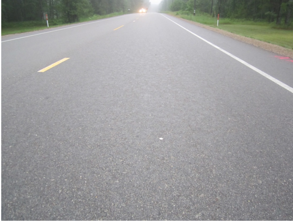
Figure 67 Advera Section at 22-Month Inspection in Rapid River, MI
