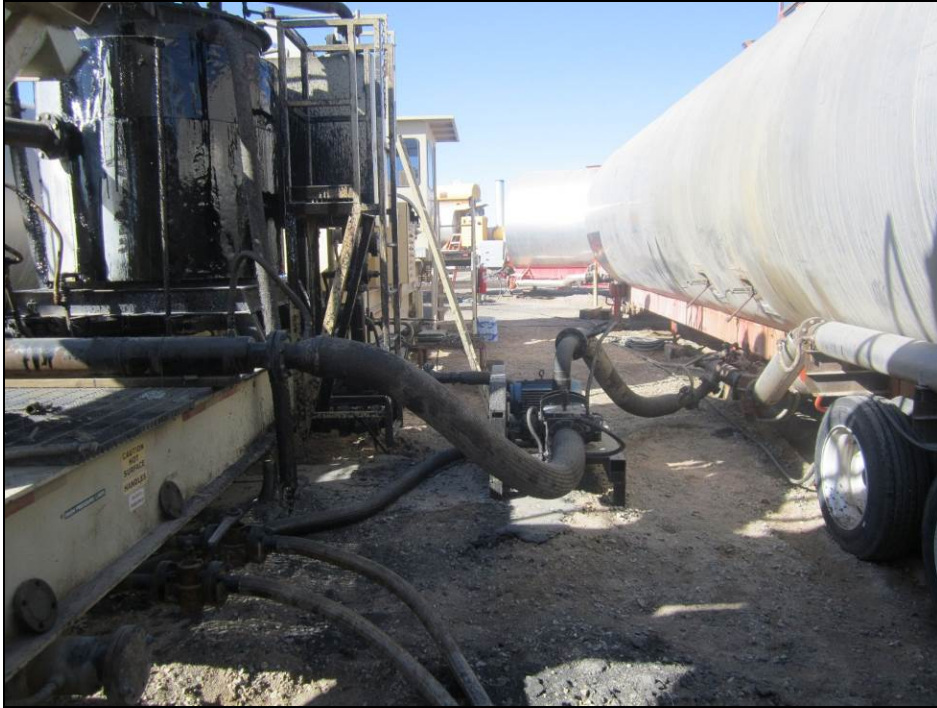
Figure 105 Tanks Used to Blend (left) and Store (right) Sasobit in Casa Grande, AZ
