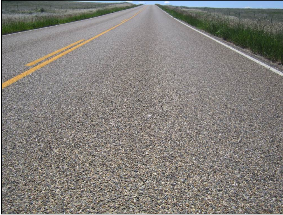
Figure 77 HMA Control Section at 22-Month Revisit in Baker, MT
