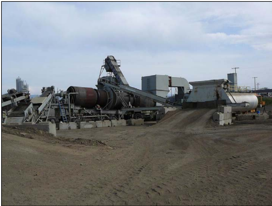
Figure 41 Granite Northwest Portable Asphalt Plant used in Walla Walla, WA
