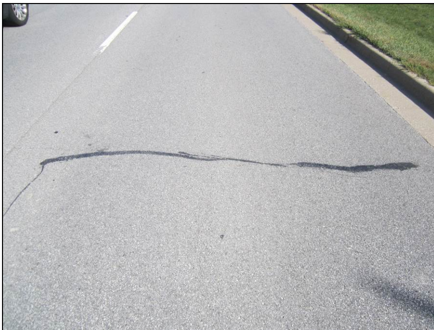
Figure 86 Example of Low-Severity Transverse Crack in Munster, IN
