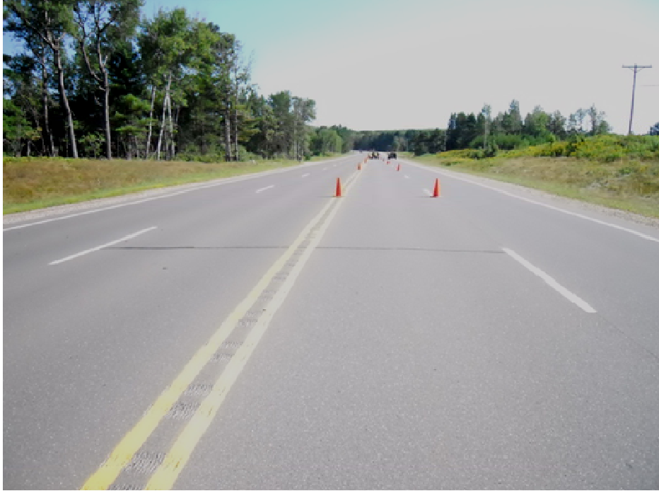
Figure 20 Transverse Cracking in WMA Section in Iron Mountain, MI
