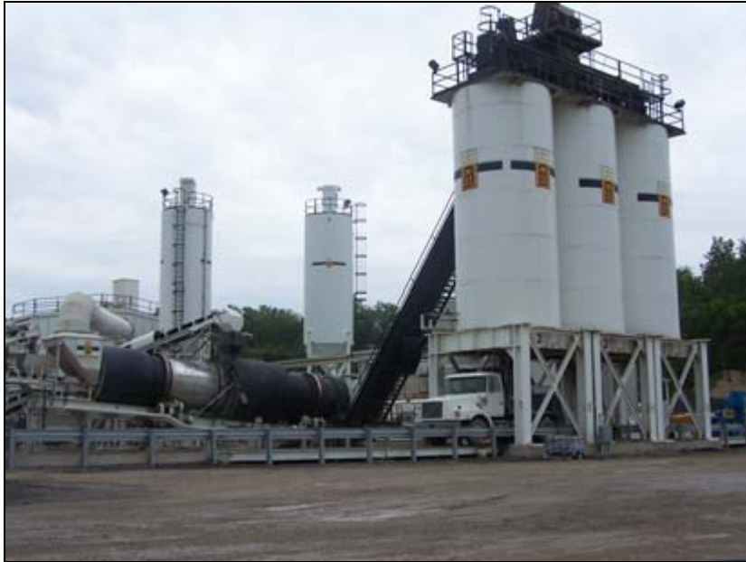
Figure 13 CMI Counter-Flow Drum Plant in St. Louis, MO (23)
