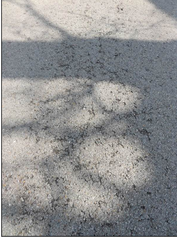
Figure 27 Fatigue Cracking in Evotherm Section in Franklin, TN
