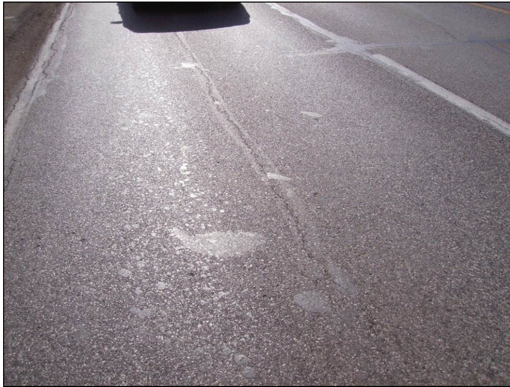
Figure 16 Example of Non-Wheelpath Longitudinal Cracking in St. Louis, MO
