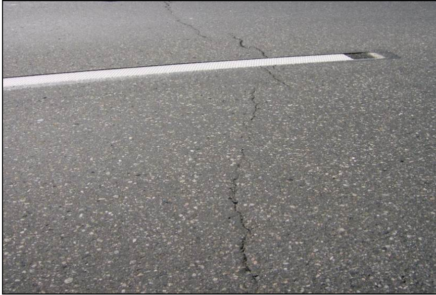
Figure 23 Transverse Cracking in WMA Section in Silverthorne, CO (24)
