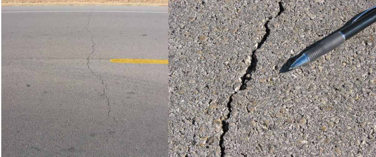
Figure 34 Photos of transverse cracks on the Graham, TX project after 30 months
