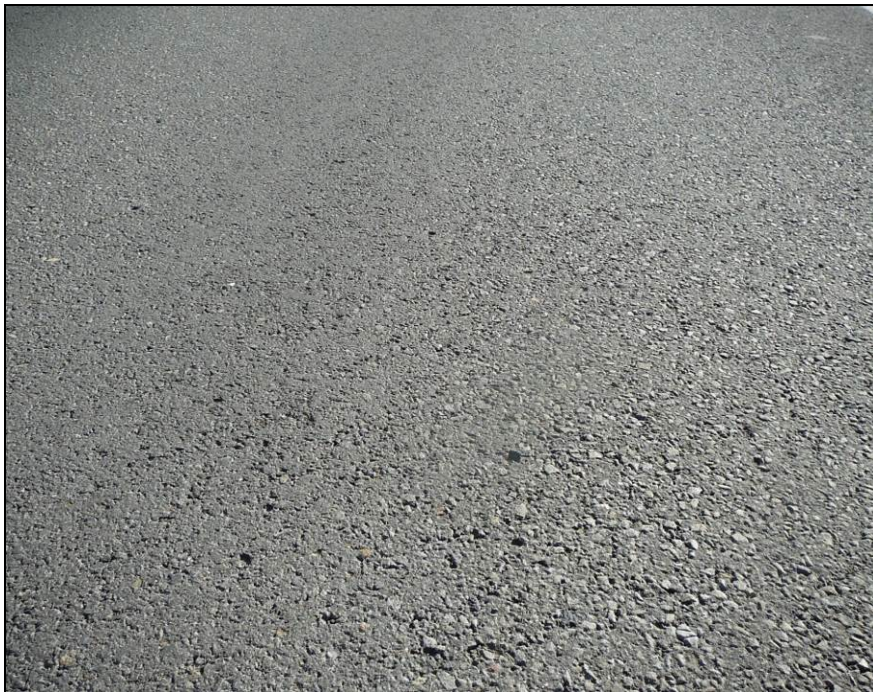
Figure 48 HMA Surface Texture at 13-Month Inspection in Walla Walla, WA
