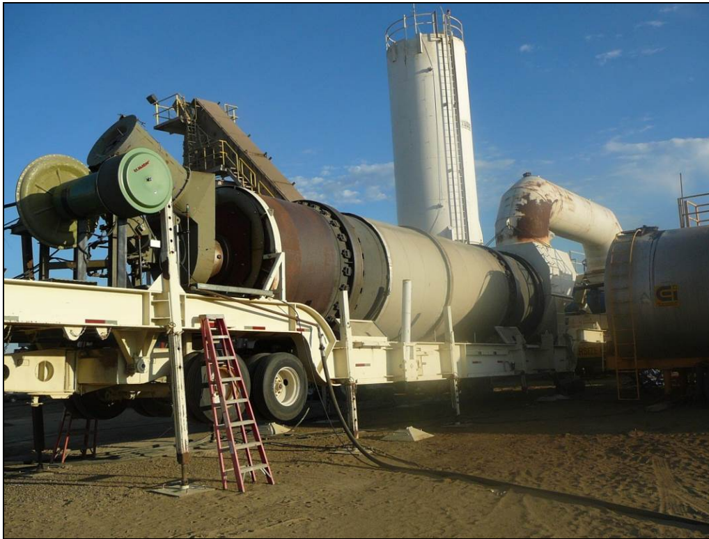
Figure 73 Portable Parallel Flow Drum Plant in Baker, MT
