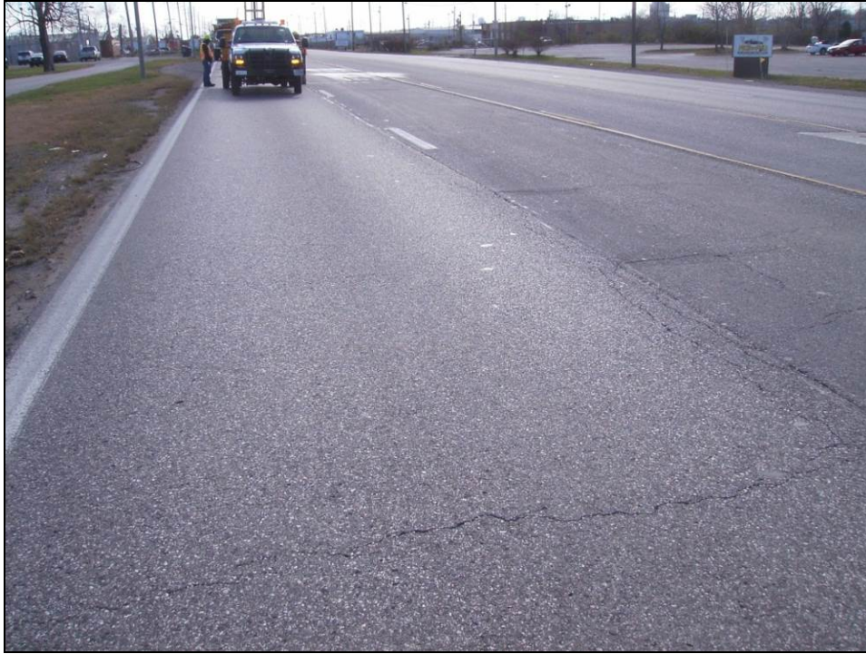
Figure 17 Example of Transverse Cracking in St. Louis, MO
