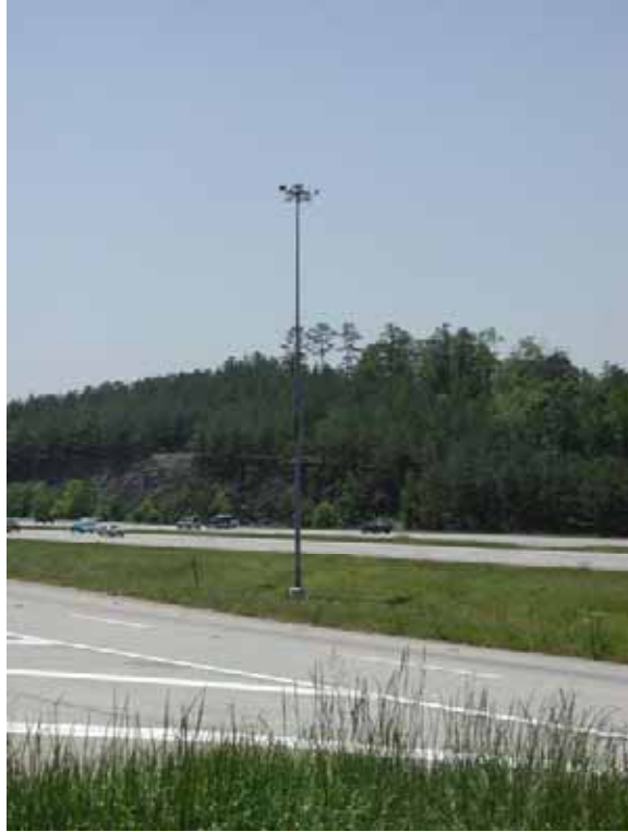
Figure 3.1. High Mast Luminaire Structure
