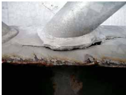
Figure 2.4. Crack Formed at the Connection of Small Diagonal Members to a Big Chord Member During Galvanizing
