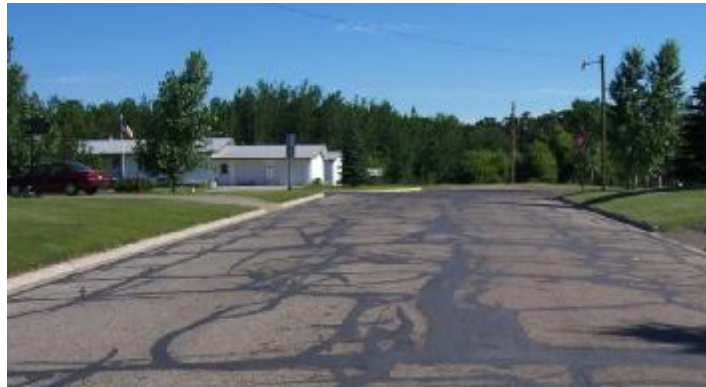
Photograph 2-2: Excessive Crack Filling (Photograph by Dale Decker)
