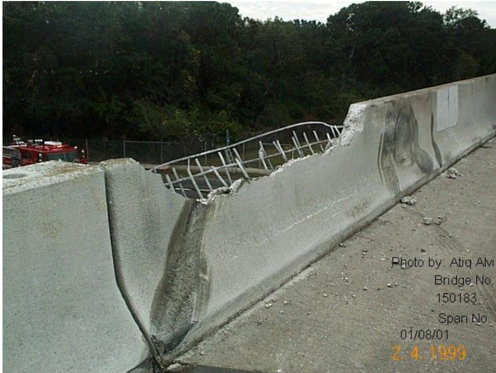
Figure 3. Damage to bridge railing, St. Petersburg, FL...
