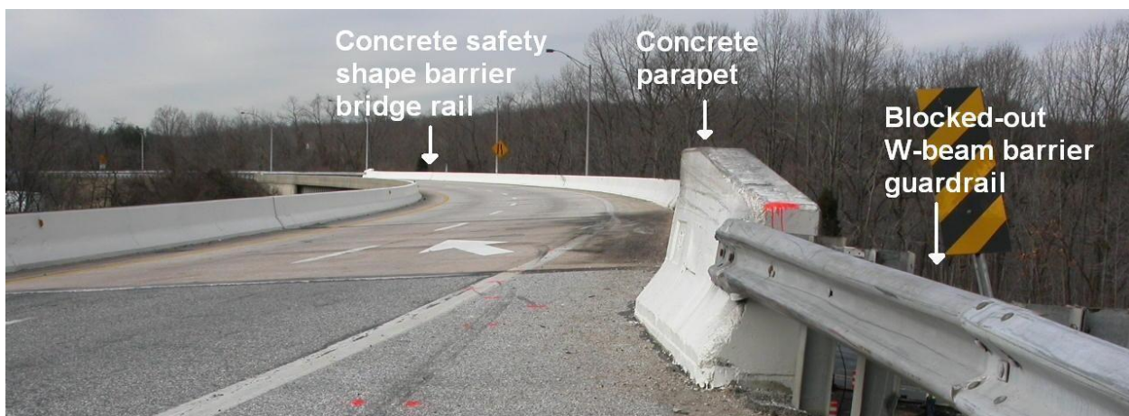
Figure 28. Crash site in Elkridge, MD where a fuel truck penetrated a concrete bridge railing. [NTSB09a]
