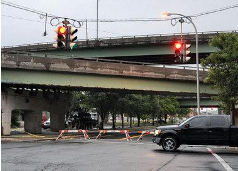
Figure 12. Site of bridge railing penetration, Syracuse, NY. [Syracuse12]
