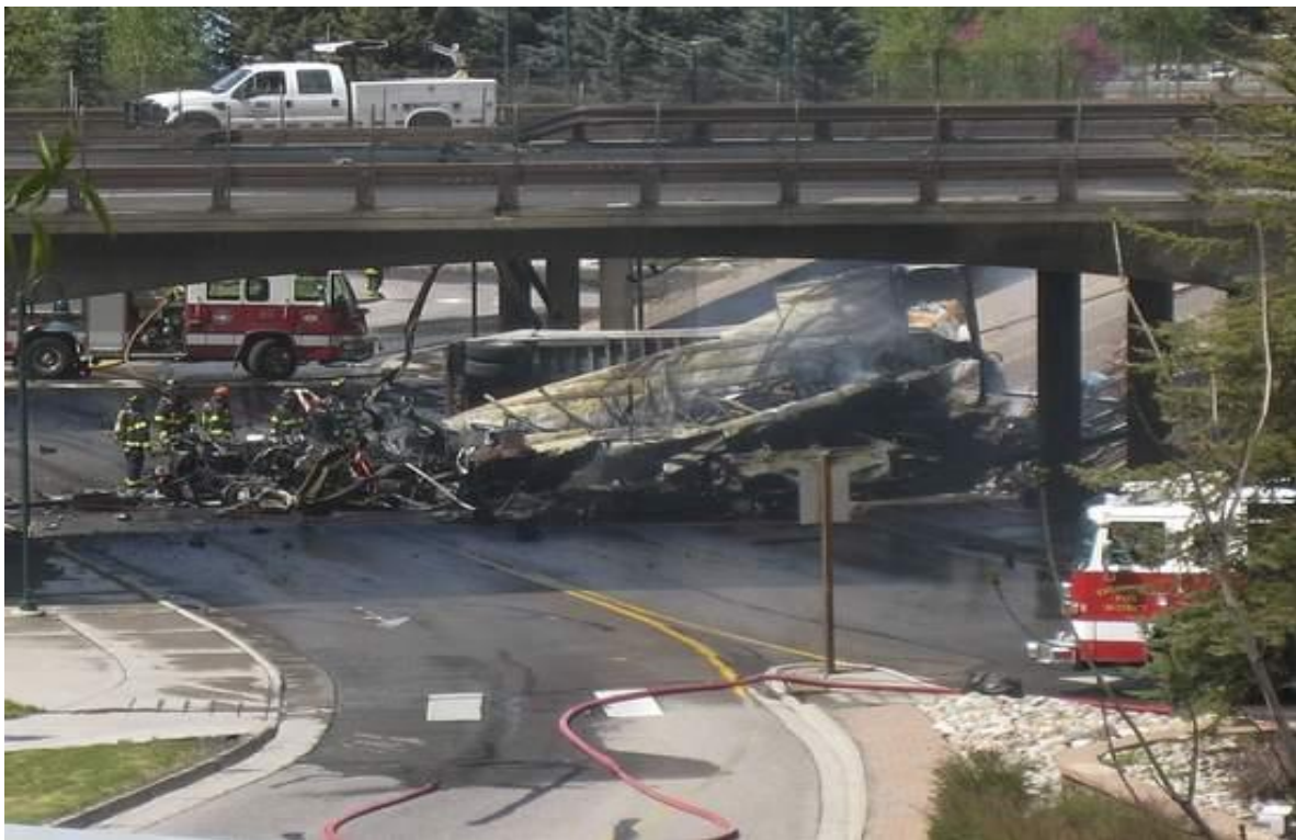
Figure 10. Damaged W-beam bridge rail and final position of truck on local road under bridge, Avon, CO. [Avon12]
