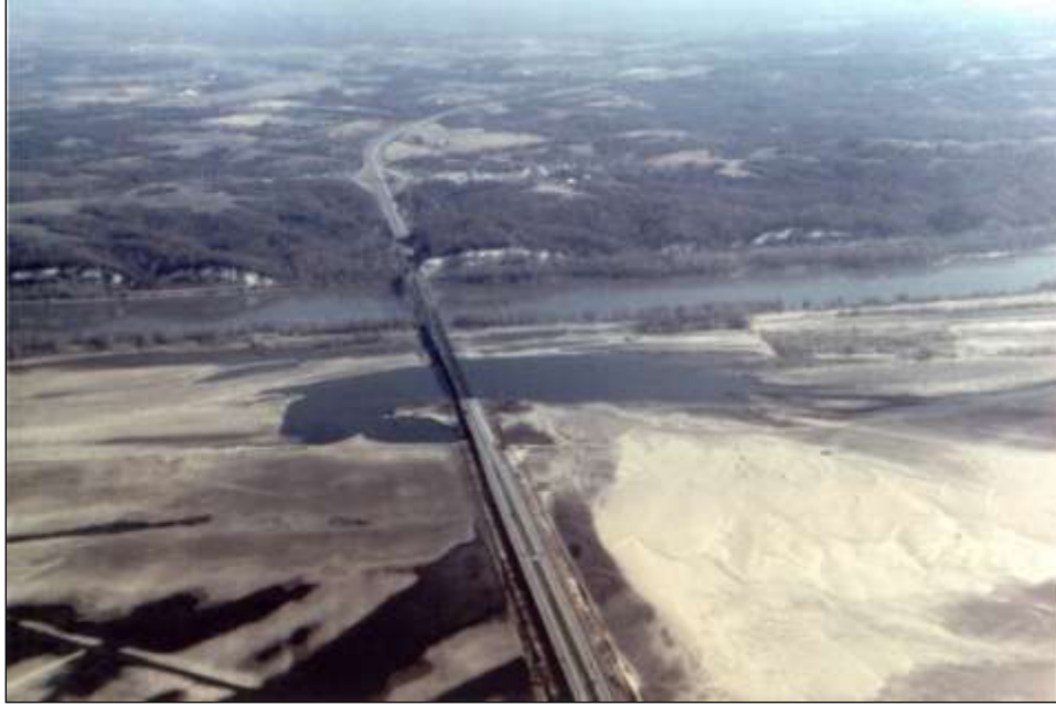
Figure 3-7. Scour Condition B at Interstate-70 Bridge over the Missouri River
