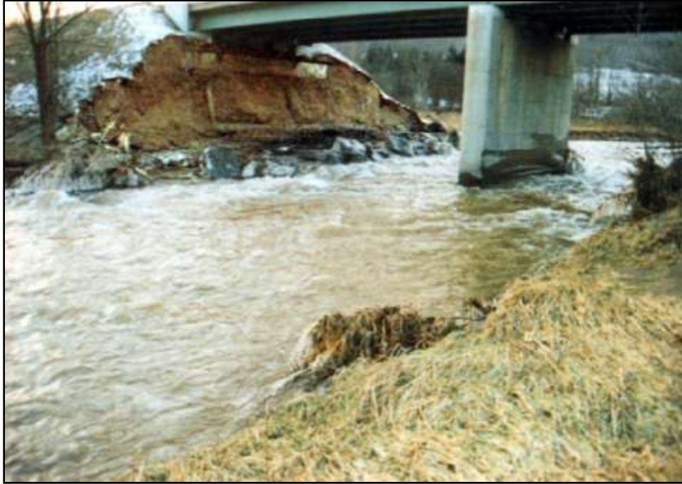
Figure 3-5. Scour Condition A led to failure of the channel bank and road embankment at this spill-through abutment
