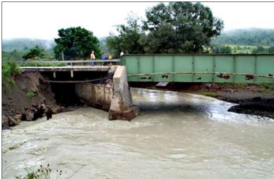
Figure 3-6. Scour Condition A led to failure of the channel bank and road embankment at this wing-wall abutment
