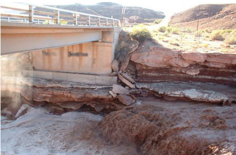
Scour can excavate soil and rocks from around bridge piers, putting the structure at risk for premature failure.
