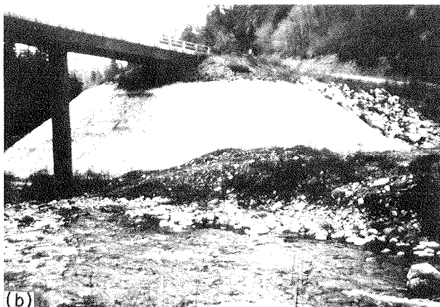
Figure B-5. Photograph of Welded Wire Wall used as bridge abutment: (a) bridge abutment under construction, (b) completed abutment.
