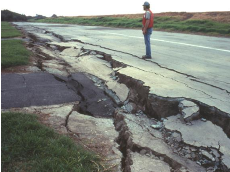
Figure 5: Roadway damaged from lateral spreading in 1989 Loma Prieta earthquake (from Nakata et al., 1990)
