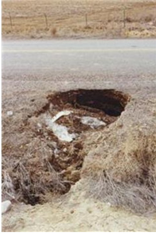
Figure 4: Road damage from a sinkhole in Colorado. Photo by Jon White.
