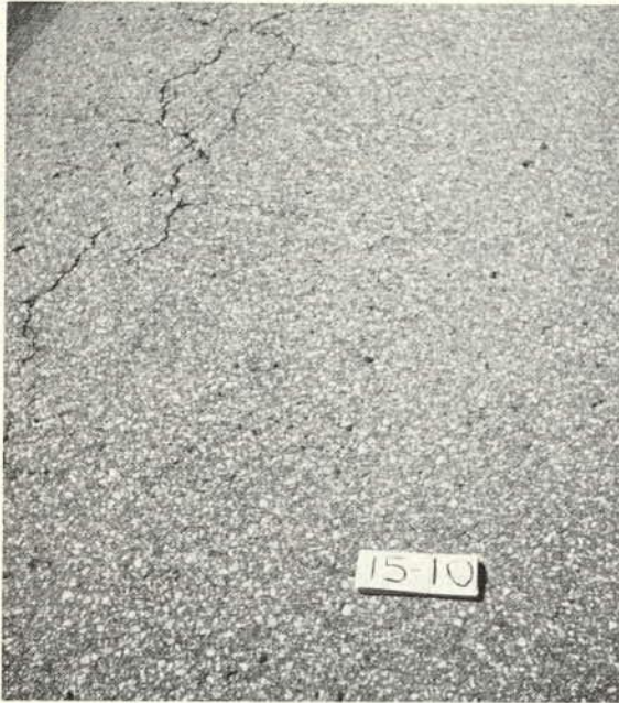
A pavement with longitudinal cracking in the wheel-path (Rating 4.0)
