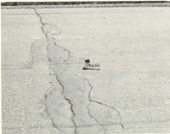
The same crack, which has progressed to moderately multiple; i. e., the associated cracks have formed into a block pattern. (Rating 3.5)
