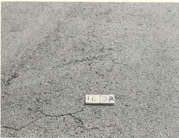
The start of random shrinkage cracking associated with weathering of the bituminous mat. (Rating 2.5)
