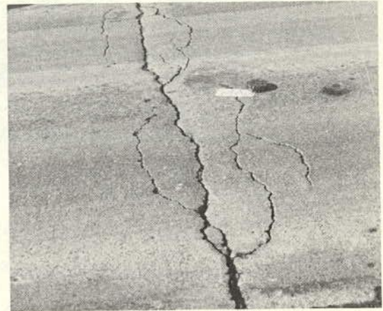
A crack that is "slightly" multiple; i.e., there are some associated cracks. (Rating 4.0)
