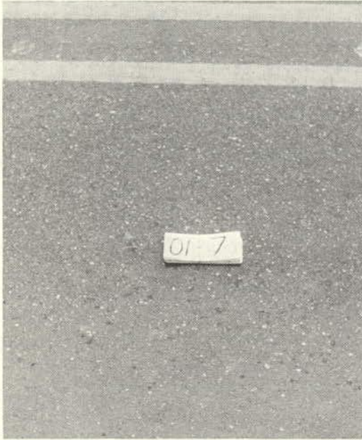
A relatively new plant-mix overlay with the aggregate showing more in the wheelpath, but not protruding. (Rating 4.2)
