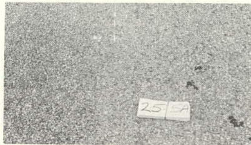
A chip seal which is just starting to get rich in the wheelpath. However, the aggregate still shows and protrudes. (Rating 4.0)
