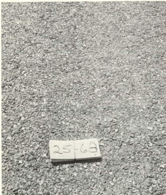
An unsealed surface mix with the coarse aggregate showing and protruding 1/16 in. and more in some cases. (Rating 2.5)
