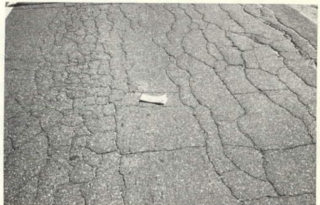
A pavement with alligator cracking in wheelpath (Rating 2.0)
