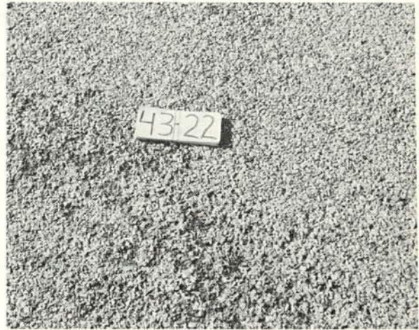
A chip seal with between 10 and 20 percent of the seal coat aggregate kicked out in the wheelpath. (Rating 3.5)
