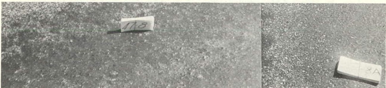
A condition where asphalt has bled up over aggregate or aggregate has been eroded off, leaving excess asphalt. (Rating 2.0)
