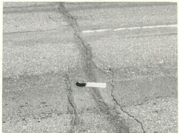
A sand seal worn off and original mat aggregate showing almost the entire length of road. (Rating 2.0)
