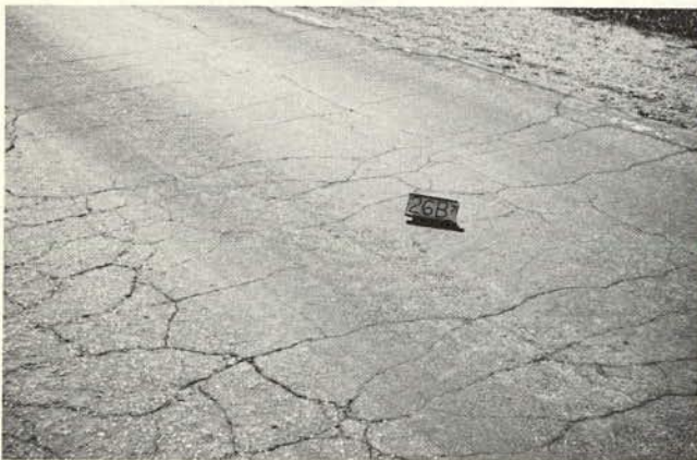
A pavement with map or block cracking in wheelpath (Rating 3.0)
