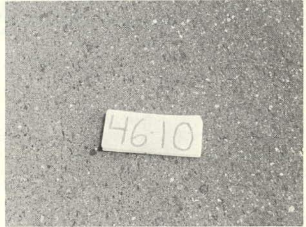
An unsealed surface mix with the coarse aggregate showing and protruding less than 1/16 in. in wheelpath. (Rating 3.5)
