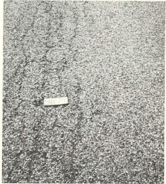
A pavement with longitudinal cracks beginning to connect (Rating 3.5)
