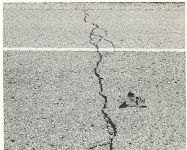
A crack open more than 1/2 in. (Rating 1.0)
