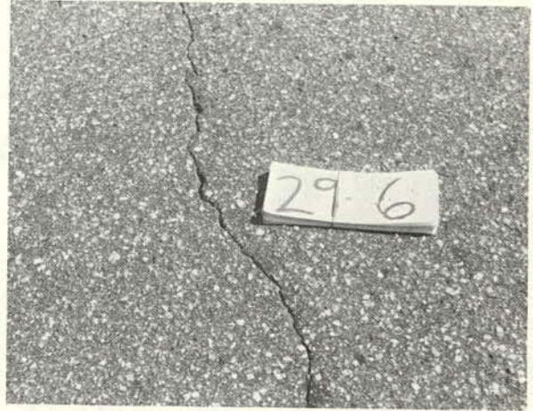
A bituminous mat in which the sand matrix is beginning to erode away between the wheelpaths exposing the coarse aggregate and making it protrude. (Rating 3.0).
