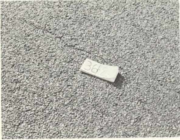
The area between the wheelpaths of this pavement appears slightly drier between the wheelpaths and a few particles have been eroded off. (Rating 4.0)
