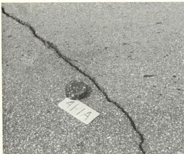
A crack open about 1/4 in. to 1/2 in. (Rating 2.0)
