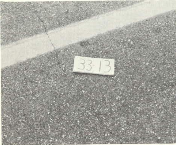
A hairline crack that is not open at all. (Rating 5.0)
