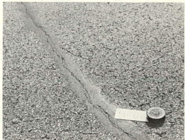
The development of random cracking in block patterns. (Rating 2.0)
