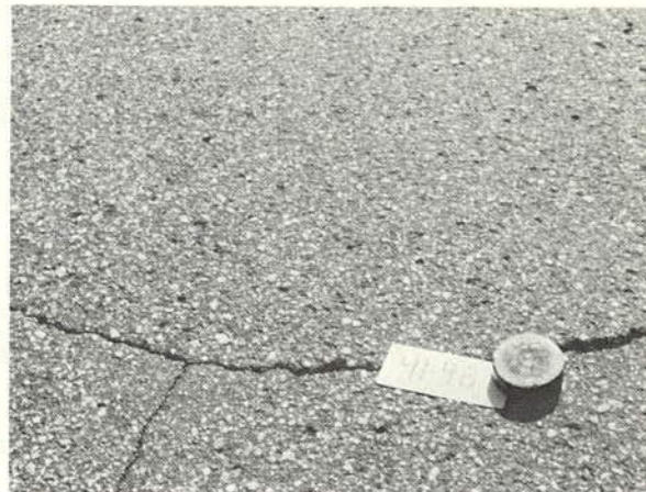
Moderate abrasion of a crack, which refers to wearing back, including some coarse aggregate particles eroded out. (Rating 3.0)
