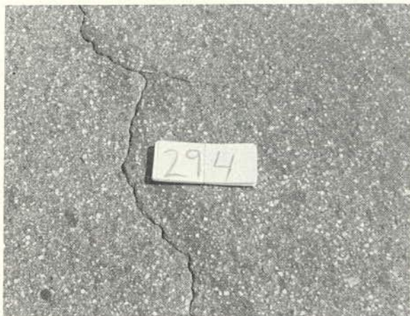
Slight abrasion of a crack, which refers to wearing back of the sand matrix. (Rating 4.0)
