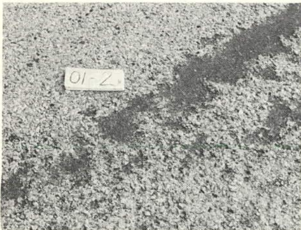
A chip seal with over 25 percent of the seal coat aggregate kicked out in the wheelpath, but bituminous material still covering original mat. (Rating 2.5)
