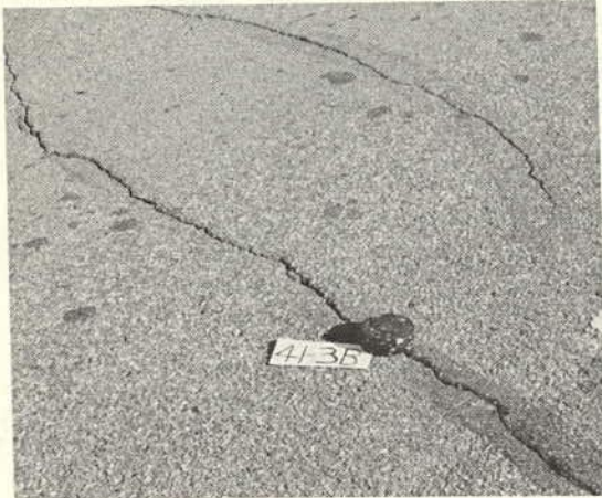
A crack that is not multiple. (Rating 5.0)
