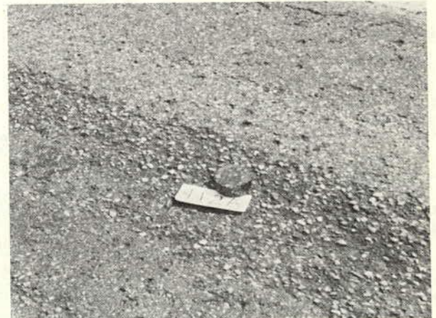
A surface which has worn in the wheelpath to the extent that the coarse aggregate is being kicked out. (Rating 1.0)
