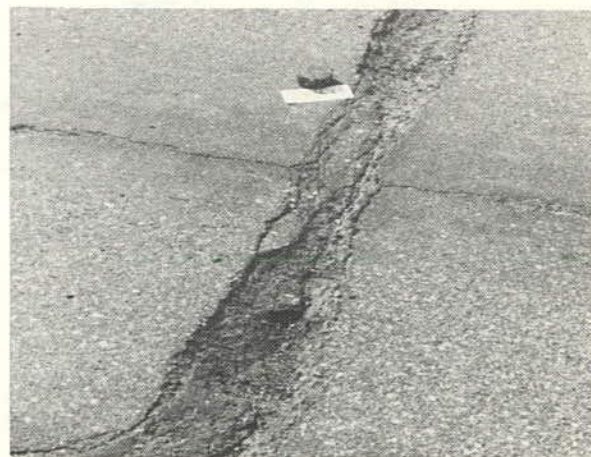
A crack that has been abraded all the way through the mat. (Rating 1.0)
