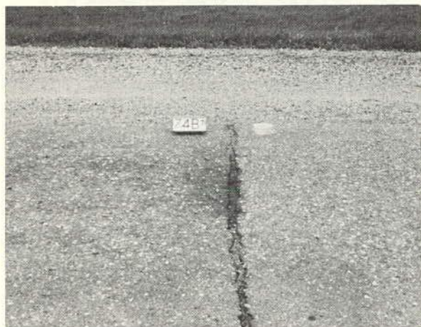
Severe erosion of a crack, which means that it is eroded more than one-half the way through the mat. (Rating 1.5)
