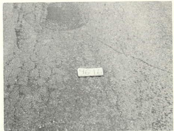
A seal coat with more than 50 percent of seal aggregate eroded off across the pavement and distress in original mat showing through. (Rating 1.5)
