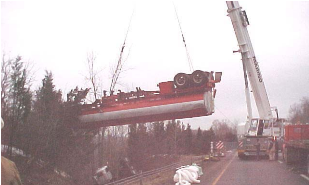
FIGURE 27 Use of a crane to remove an overturned tanker truck. (Courtesy: Connecticut DOT.)
