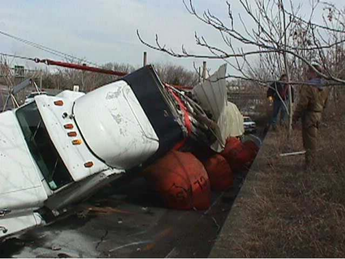
FIGURE 26 Air-cushion recovery system righting an overturned, fully loaded semi-tractor trailer. (Courtesy: New Jersey DOT.)
