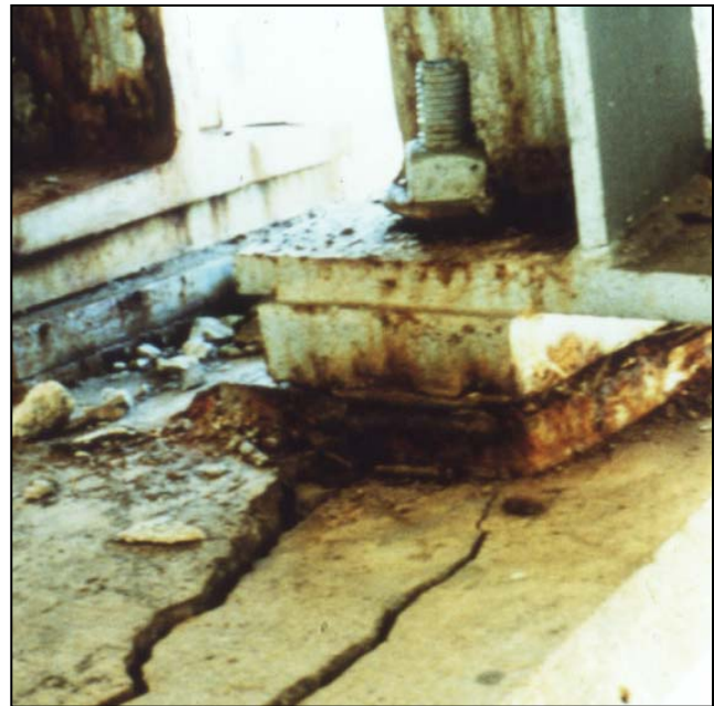
FIGURE 19 Frozen bearing and damaged bridge seat under joint.
