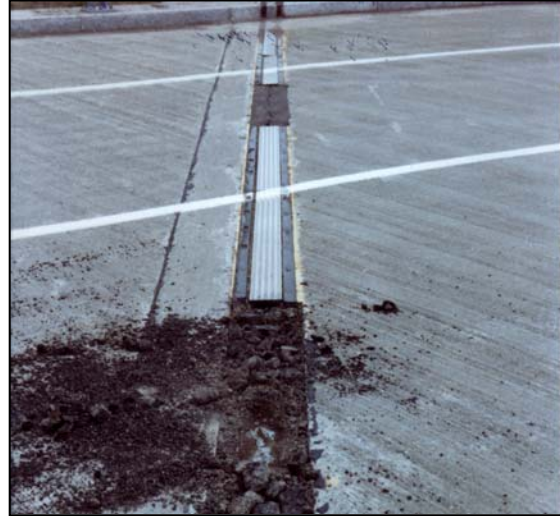
FIGURE 33 Damaged cushion seal.
