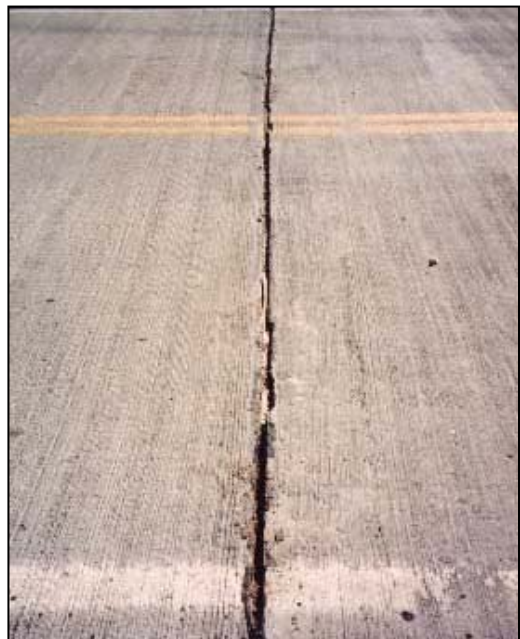
FIGURE 23 Damaged poured-in-place seal.
