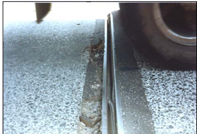
FIGURE 29 Damaged strip cell.
