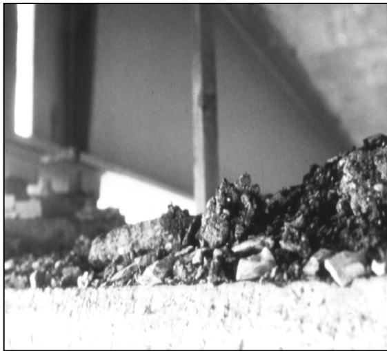
FIGURE 16 Debris on bridge cap.
