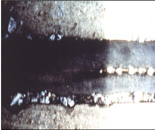
FIGURE 21 Debris lodged in joint seal.
