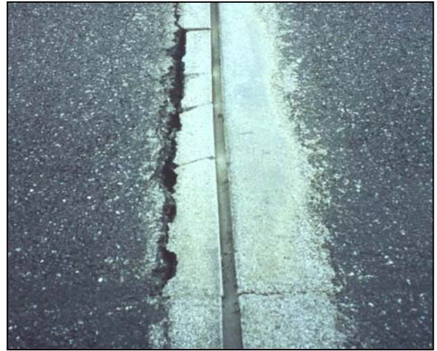
FIGURE 42 Effect of poor quality blockout material.
