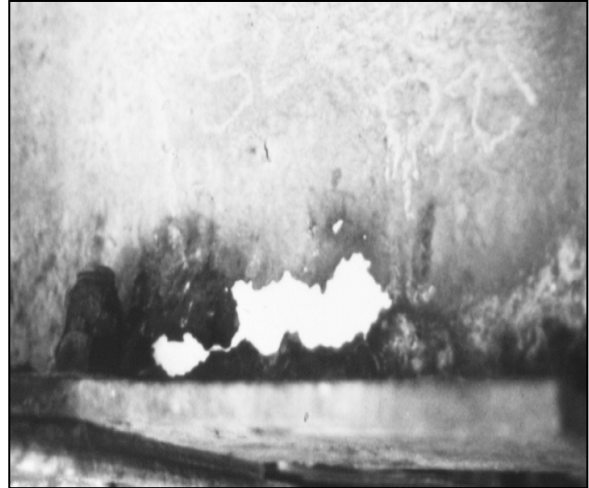
FIGURE 18 Corroded steel beam end.
