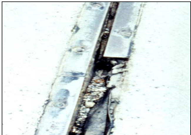
FIGURE 12 Damaged joint armor.
