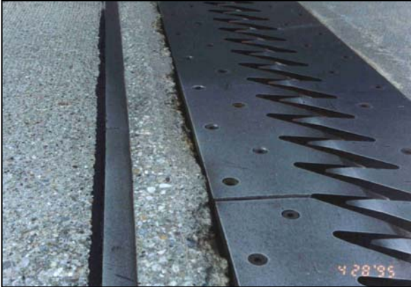
FIGURE 15 Damaged concrete around finger joint.
