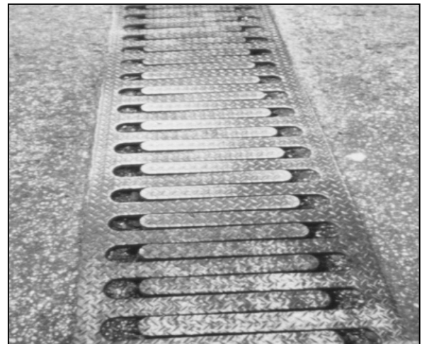
FIGURE 14 Damaged finger joint.
