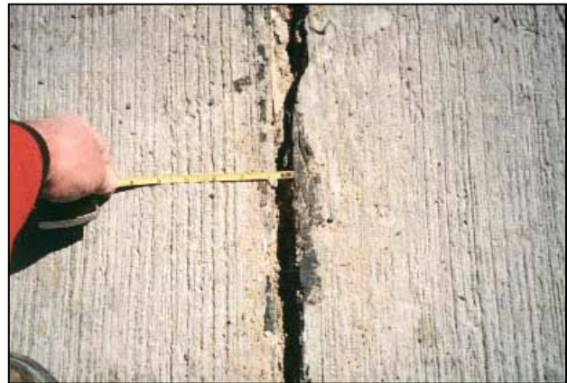
FIGURE 11 Butt joint with damaged edge.
