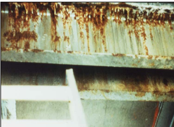
FIGURE 17 Corroded steel diaphragms under joint.
