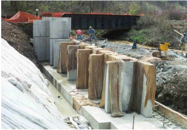
FIGURE 34 View of counterfort abutment system for a single-span bridge over Miller's Run Creek in southwestern Pennsylvania. [Source: Scanlon et al. (26).]
