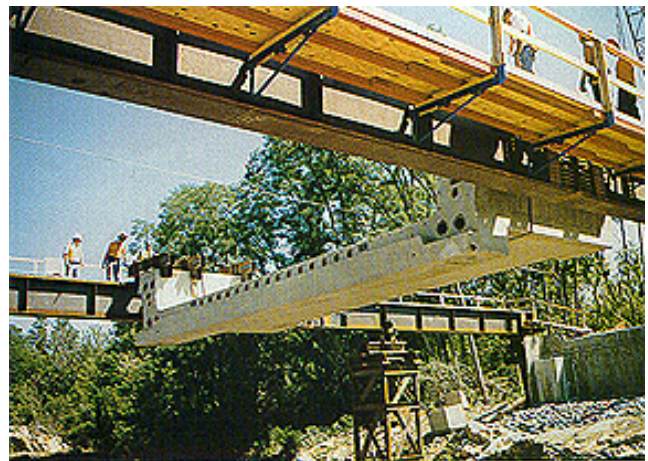
FIGURE 4 Installation of the first two channel segments of the Carpenter Road Bridge. (Source: http://www.tfhrcc.gov/pubrds/septoct98/channel.htm .)
