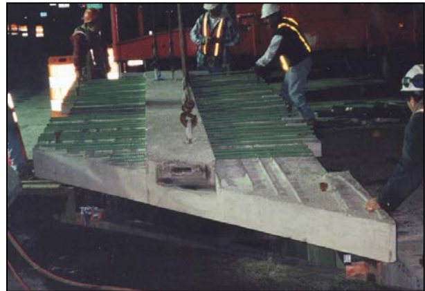
FIGURE 29 Installation of new panel of bridges at Route 7 over Route 50, Fairfax, Virginia. [Source: Babaei et al. (1).]
