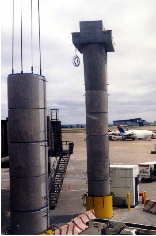
FIGURE 17 Dallas/Fort Worth International Airport people mover under construction. (Source: www.aashtotig.org ; courtesy: STOA/Carlos + Law, AE.)
