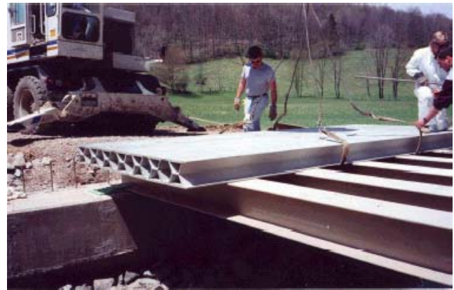
FIGURE 48 Placement of FRP deck modules over FRP stringers (Laurel Lick Bridge). [Source: Shekar et al. (34).]
