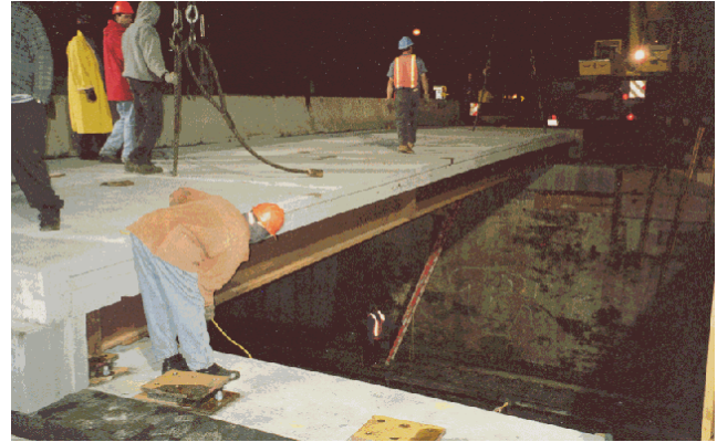
FIGURE 14 Main Street over Metro North Railroad. (Source: www.aashtotig.org ; courtesy: New York State DOT.)
