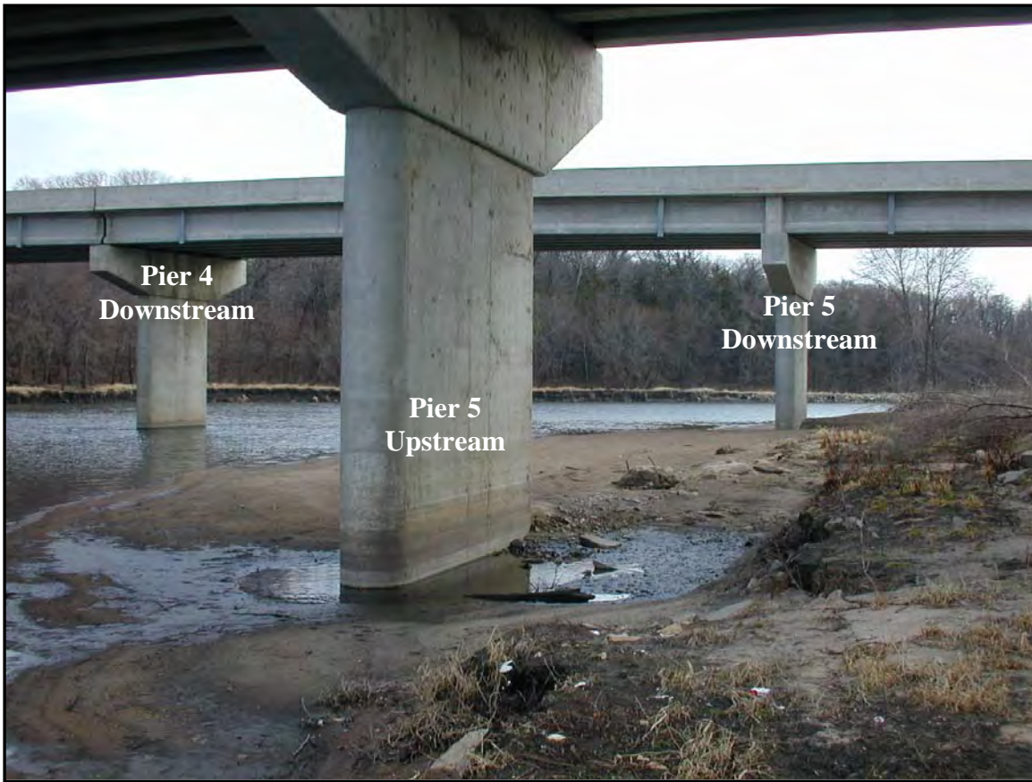
Figure 13. Looking downstream at right overbank and Pier 5 of US 218 bridge over Cedar River during low flow, 8/10/99.
