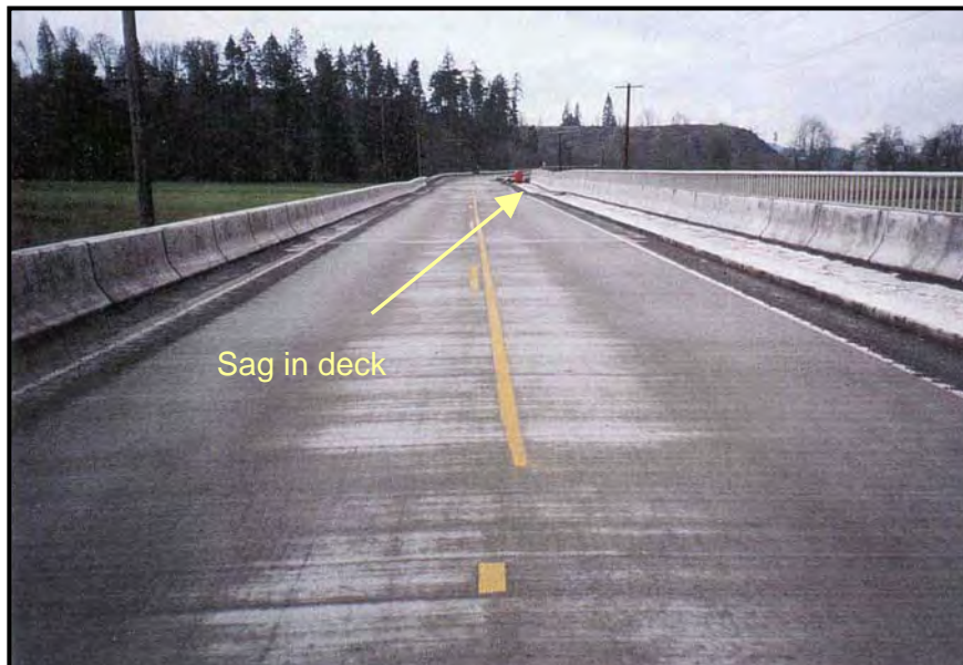
Figure 10. Looking west toward sag in bridge deck due to failure of pier #9 during the February 1996 flood.
