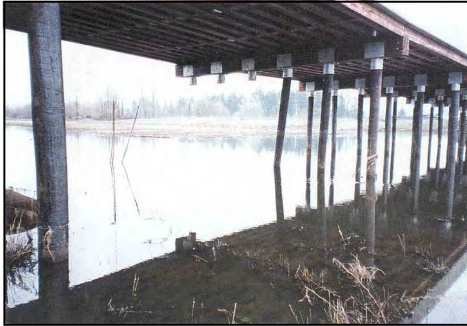
Figure 9. Looking east at failed pier #9 following the February 1996 flood.
