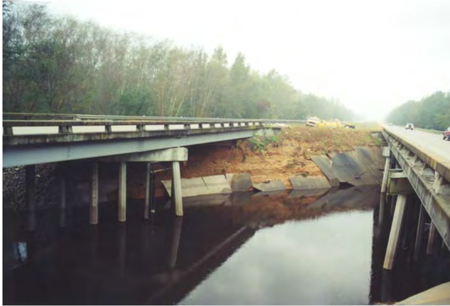
Figure 7. Looking at the east abutment from the top of the west abutment.
