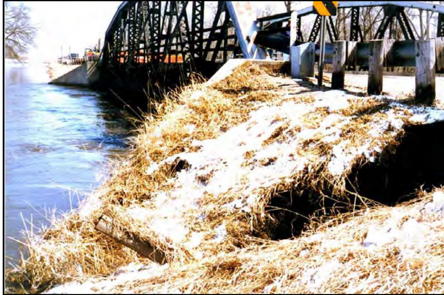
Figure 5. Looking at the upstream U.S. 12 bridge face from right bank during the April, 1997 flood.
