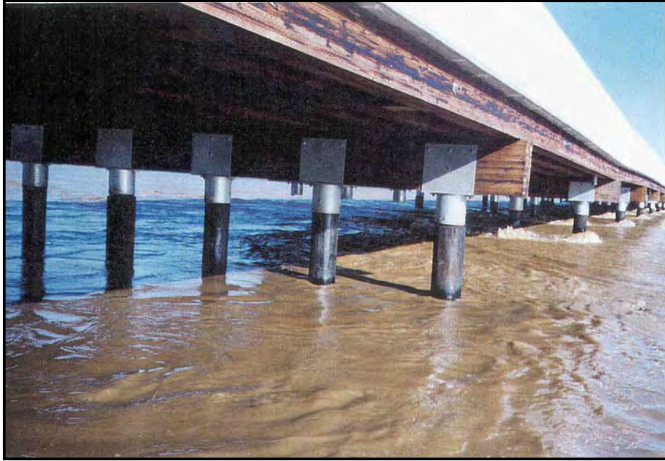
Figure 5. Looking east at Pier 10 (foreground) and Pier 9 (the pier that failed) of Galvin Road Overflow Bridge, 2/9/1996.
