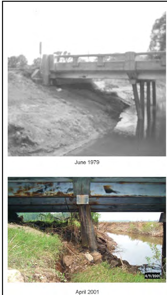
Figure 7. Looking downstream through the S.R. 35 bridge opening at left abutment and pile bent no. 2 following the 1979 and 2001 floods on Conehoma Creek.
