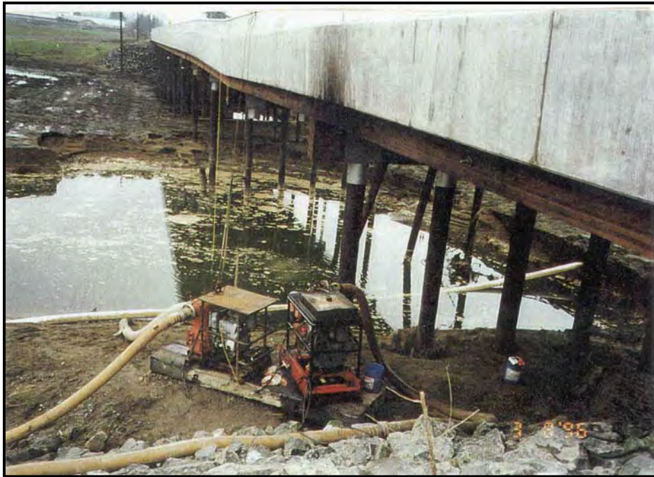
Figure 6. Looking east along downstream side of Galvin Road overflow bridge into scour hole during dewatering.
