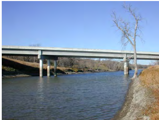
Figure 12. Post-flood conditions, looking upstream at S.R. 37 bridge from right bank
