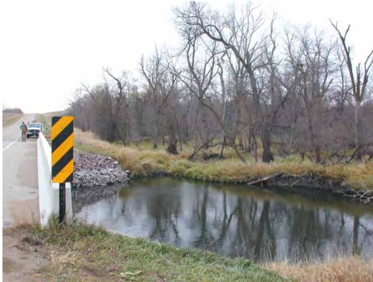
Figure 6. Looking at scoured area on right upstream bank of County Route 22, during low flow.
