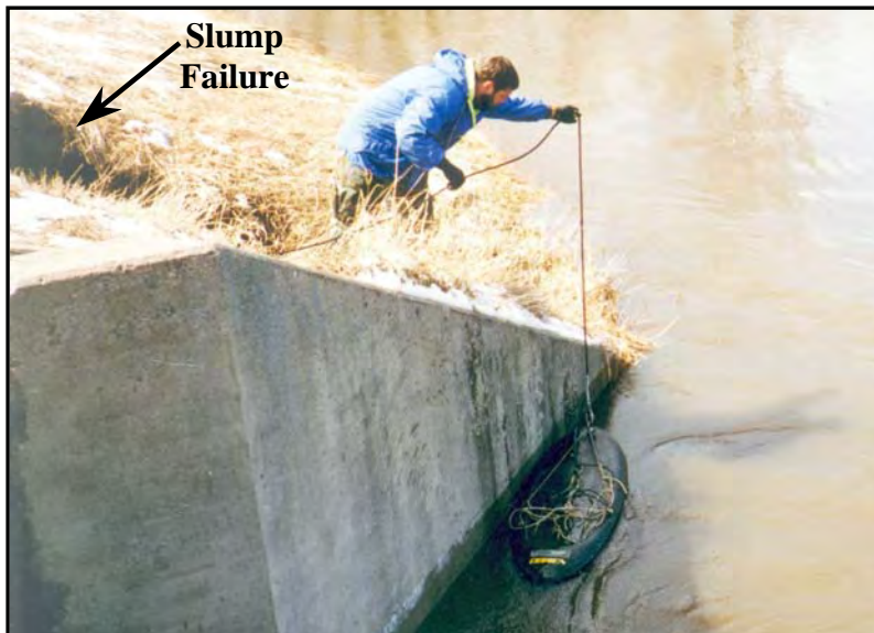
Figure 6. Scour measurement at upstream right wingwall of U.S. 12 bridge over the Pomme De Terre River; notice slump failure of embankment.
