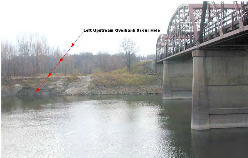
Figure 6. Looking at left upstream overbank scour hole (inside what appears to have been a much larger scour hole) from right bank along the upstream bridge face of S.R. 25 over the Minnesota River during low-flow.
