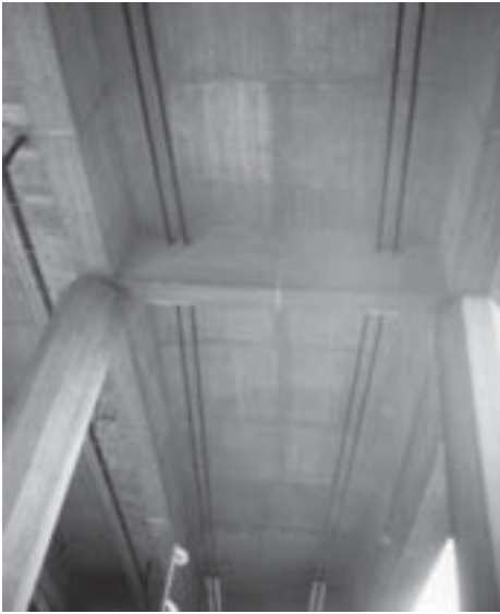
Figure 2. External longitudinal tendons have been retrofitted to the underside of a post-tensioned concrete girder near Cologne, Germany.
