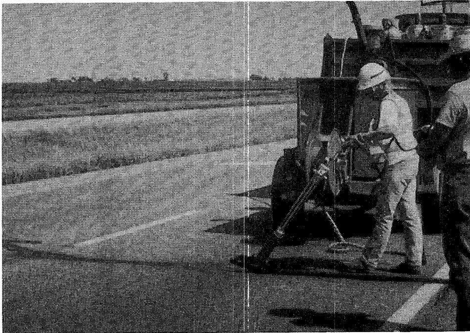
Figure 18. Hot compressed-air lance
