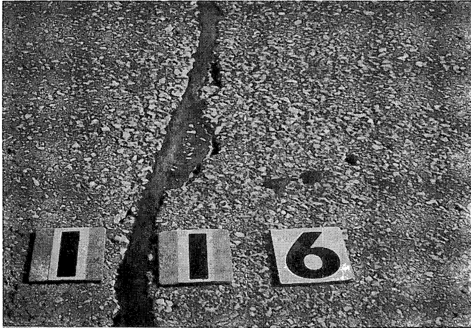
Figure 32. Typical spall and secondary crack adjacent to 890-SL seal
