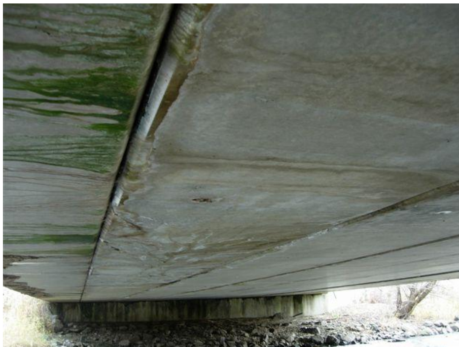
Figure 26. Example of adjacent box girder deterioration due to moisture effects
