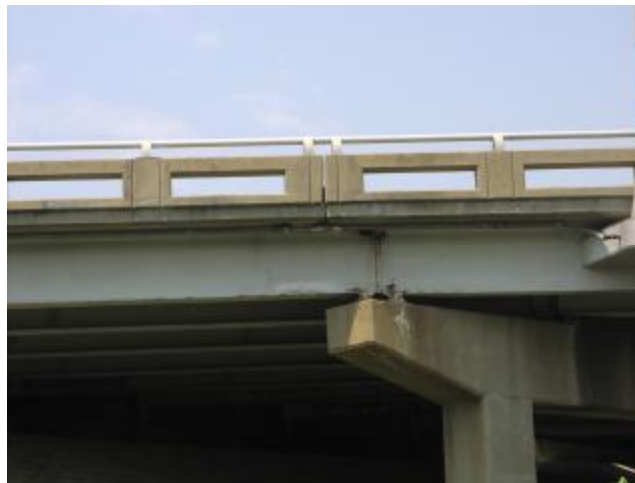
Figure 48. Deterioration of bridge due to leakage from a joint
