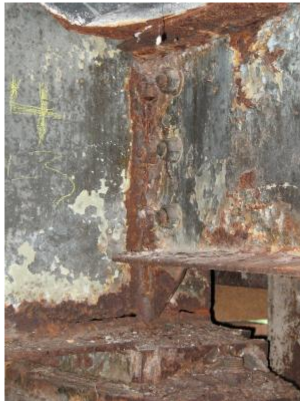
Figure 18. Corrosion at a connection of a steel bridge
