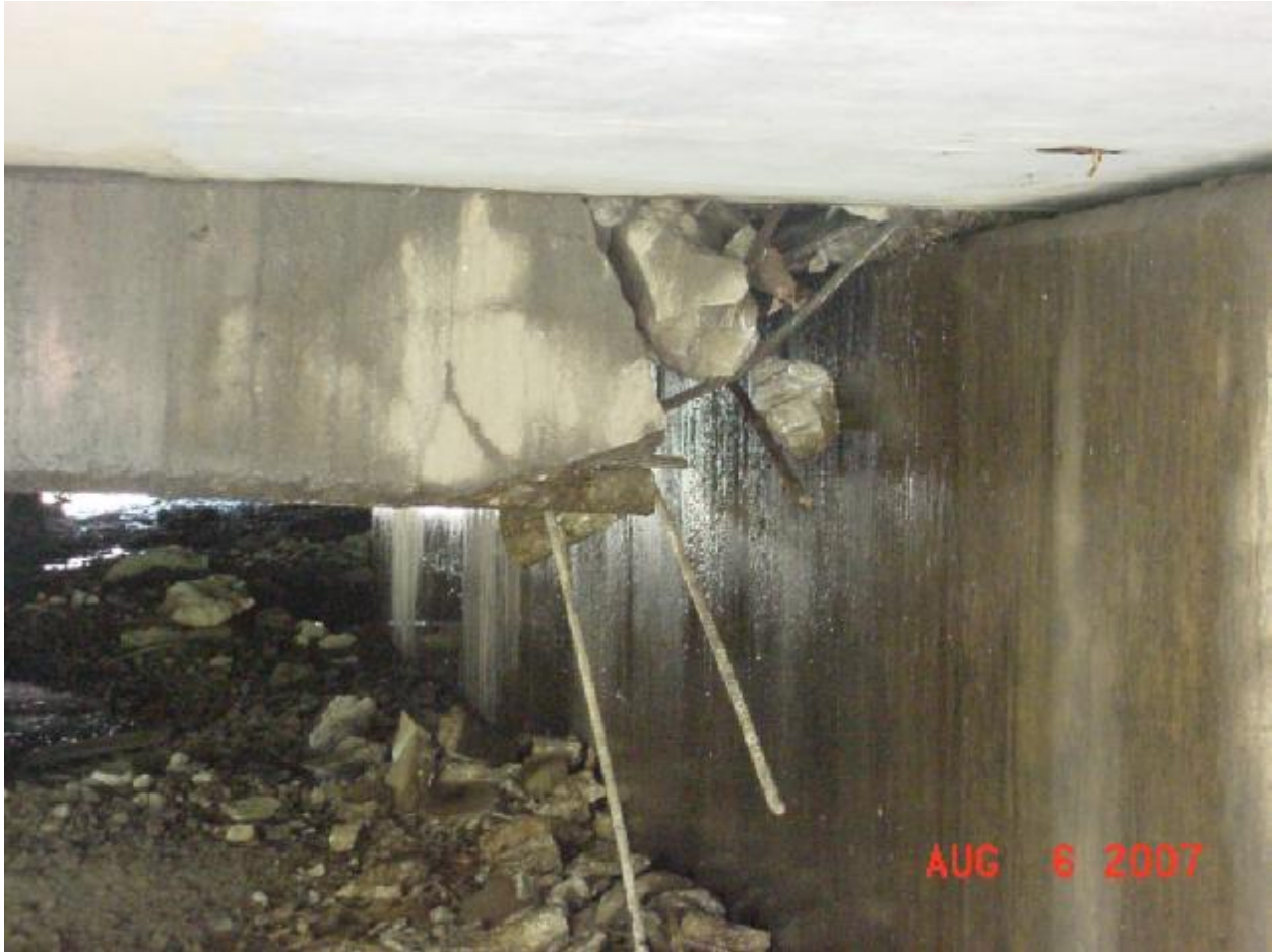
Figure 28. Failed interior girder of an adjacent box-girder railroad ridge (August, 2007)
