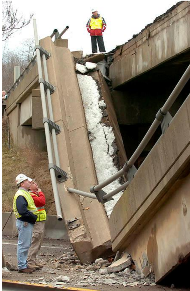
Figure 27. A collapsed exterior girder in an adjacent box-girder bridge (December, 2005)
