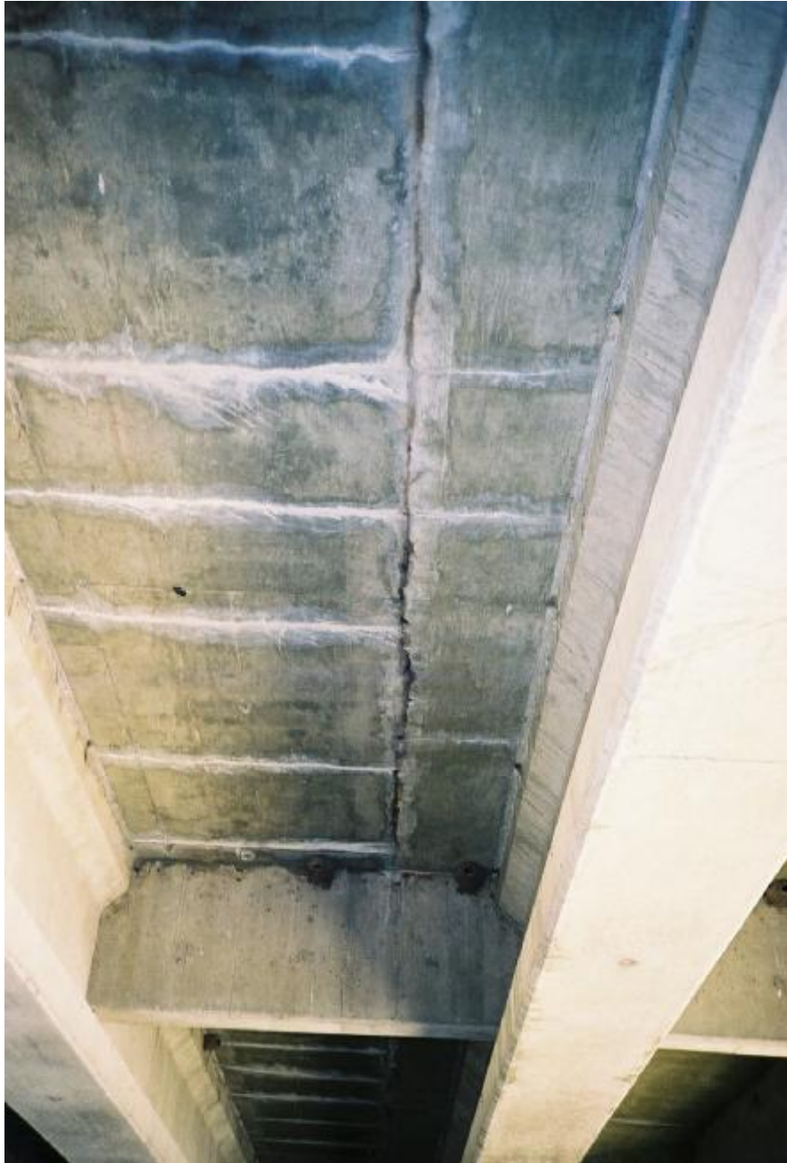
Figure 31. The condition of a phase-constructed bridge. The photo shows water seeping through the longitudinal cracks located at the interface of Phase I and Phase II. Additionally, closely spaced transverse cracks are also formed in the Phase II portion (Photo by Azizinamini).
