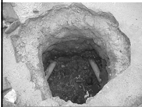
3 conduits interfere with 36" pole footing diameter
