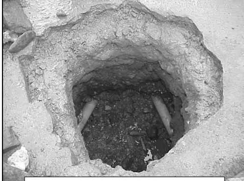
3 conduits interfere with 36" pole footing diameter
