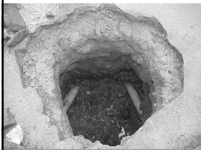
3 conduits interfere with 36" pole footing diameter
