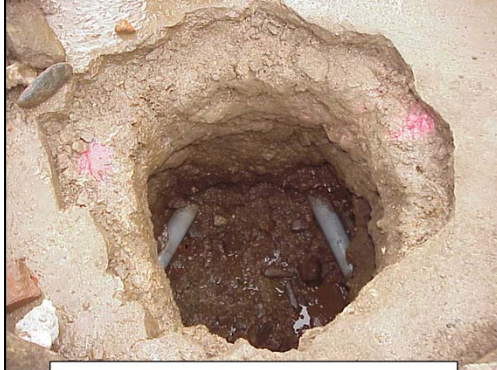
3 conduits interfere with 36" pole footing diameter
