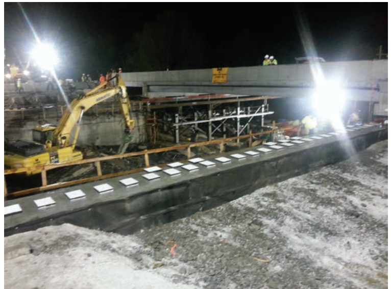
Rapid renewal methods include bridge slide techniques used on the Dingle Ridge Road Bridge project on I-84 in New York, which replaced the bridge in two weekend nights. (photo from HNTB)
