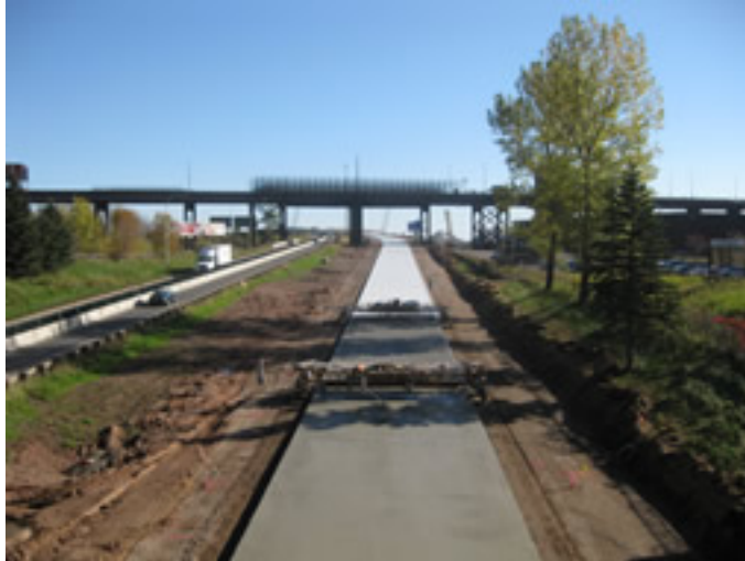
Figure 55. New Pavement Construction of a Divided Highway, Contra-Flow Operations on Other Side of Median (3)
