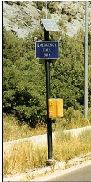
Figure 92. Call Box Mounted on Sound Barrier (1)
