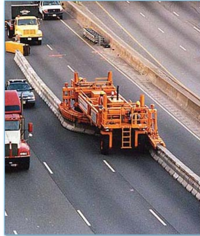
Figure 5. Moveable Traffic Barrier (1)
