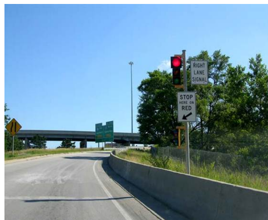
Figure 78. Ramp Metering Installation (right-lane signal) (1)
