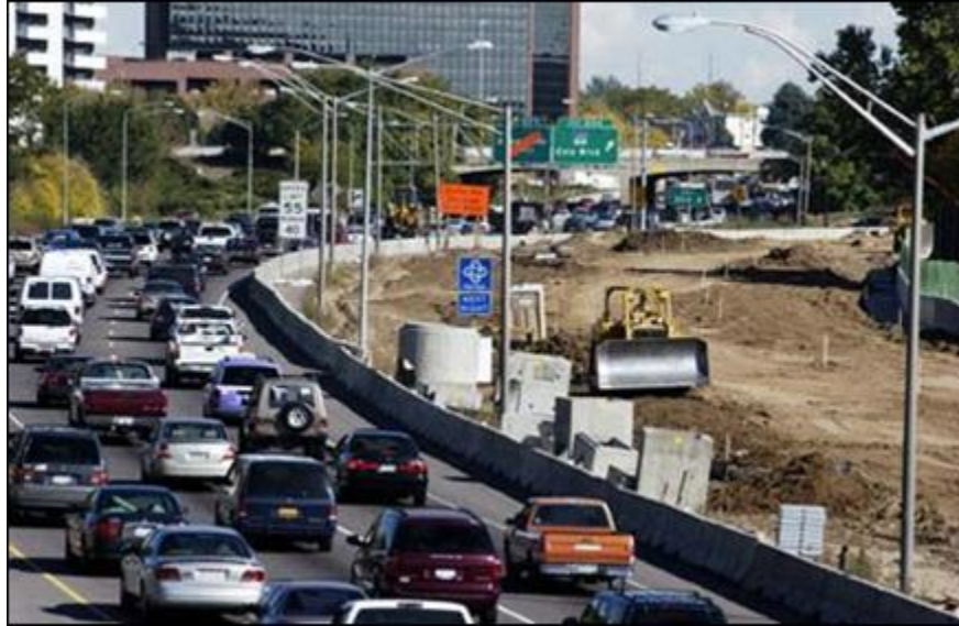
Figure 40. Construction Project Causing Freeway Congestion (1)
