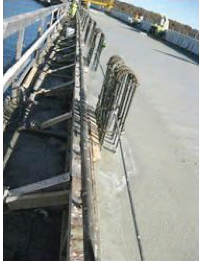
Figure F.4. Water ponding along the edge and hand finishing.
