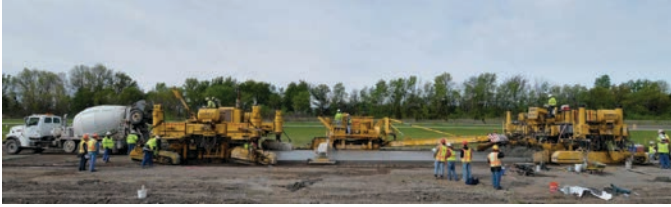
Figure 2.15. Paving train constructing R21 test sections along I-94 at MnROAD (from left to right: the mixer truck, first paver, belt placer, and second paver).
