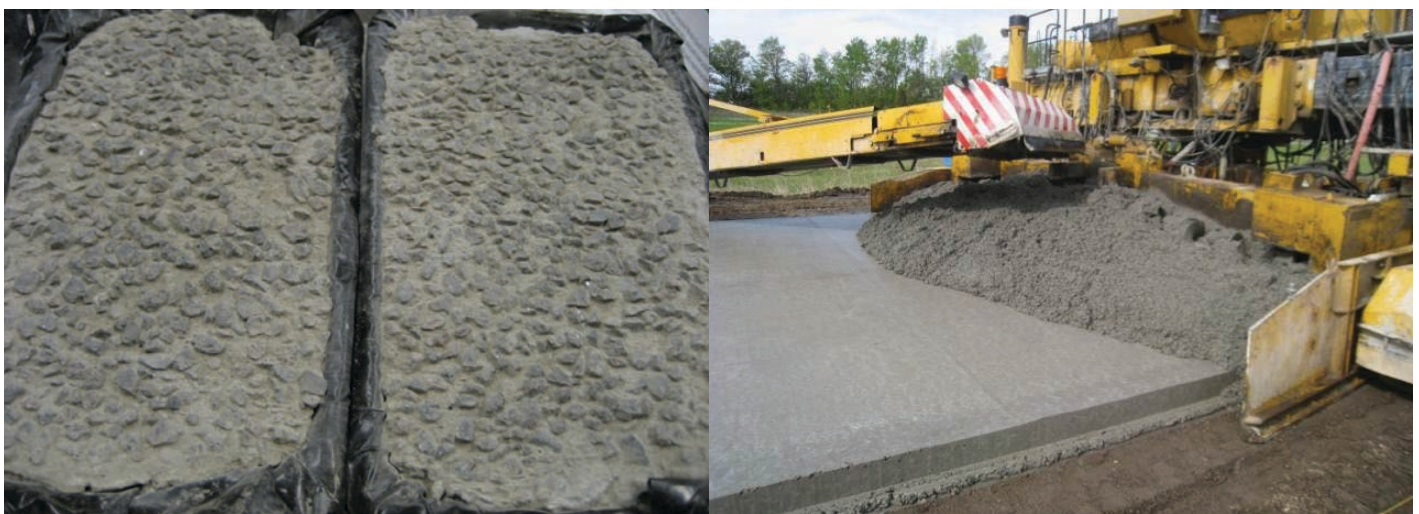
Figure 2.19. At left, PCC specimens cast in preparation for the paving and brushing of the PCC/PCC demonstration slab; at right, top-surface PCC mix being placed in front of the second paver on-site at MnROAD.
