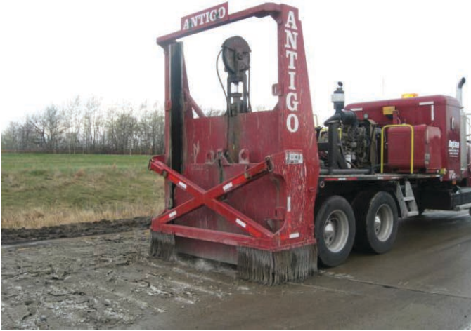
Figure 2.5. Guillotine crusher breaking existing concrete for recycling into the lower PCC layer of the PCC/PCC composite pavement.
