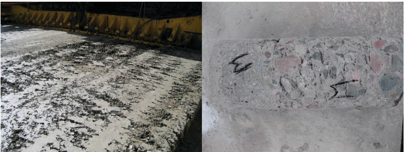
Figure 2.16. At left, “torn” edges and surface caused by concrete setting on various parts of the paver. At right, coring showed poor mix consolidation in the lower PCC at select locations.
