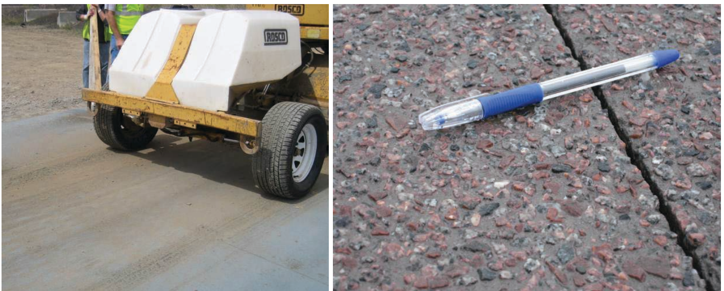
Figure 2.24. Surface after first pass with brush (left). Finished EAC surface (after wash) (right).
