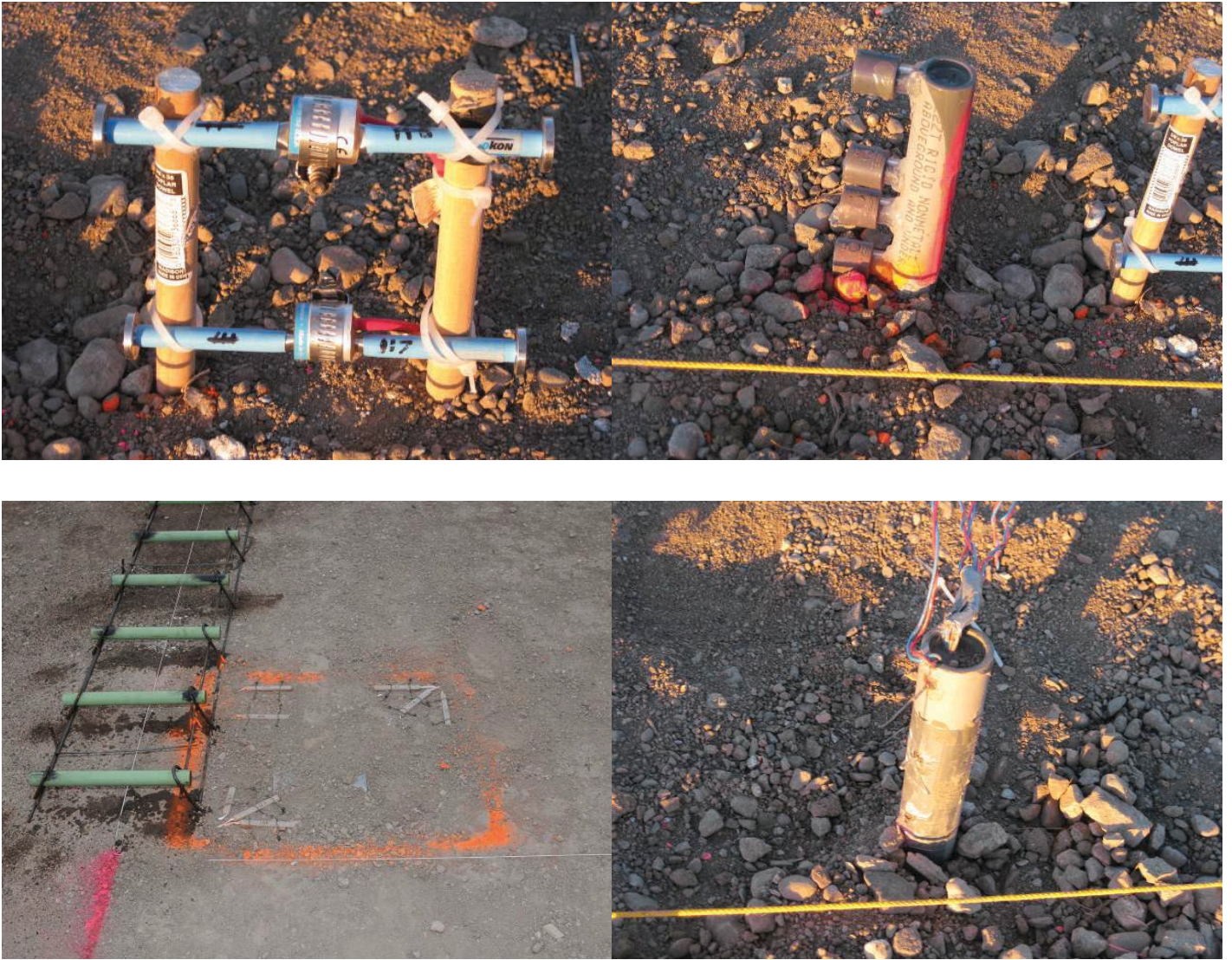
Figure 2.13. Instrumentation installed prior to placement of the PCC to measure pavement responses to temperature and traffic loads (static strain gauge, top left; dynamic strain gauges, bottom left; humidity sensors, top right; temperature sensors [thermocouple tree], bottom right).
