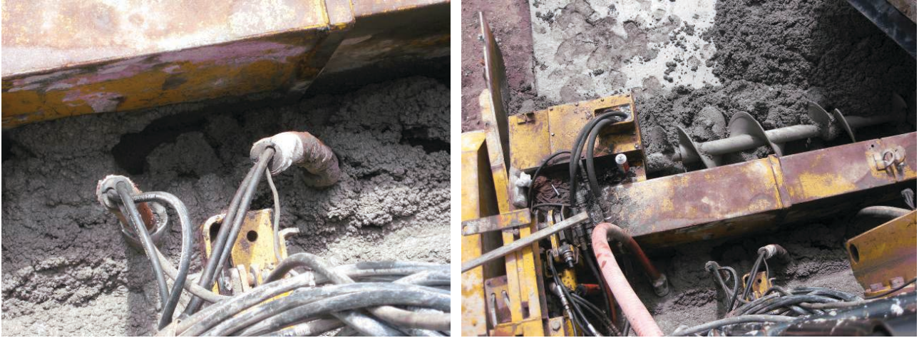
Figure 5.5. Vibrating the upper lift PCC and edge of upper lift paver relative to the lower PCC layer.
