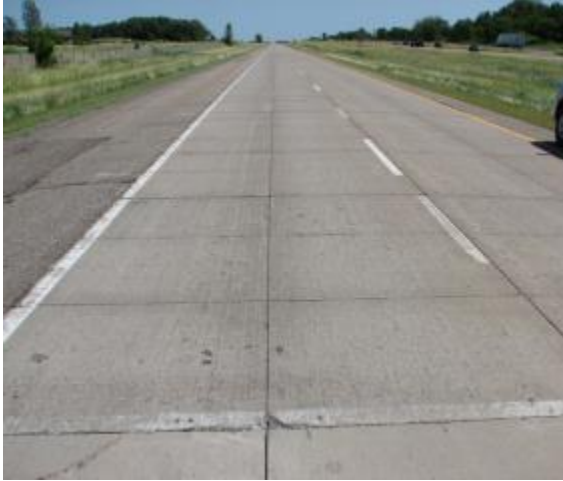
MnRoad Cell 96. Bonded concrete overlay 6 in. thick with a 5 ft by 6 ft joint spacing without dowels. Performance: no cracked panels but noticeable faulting has occurred. Will be diamond ground in 2011 to improve ride.
