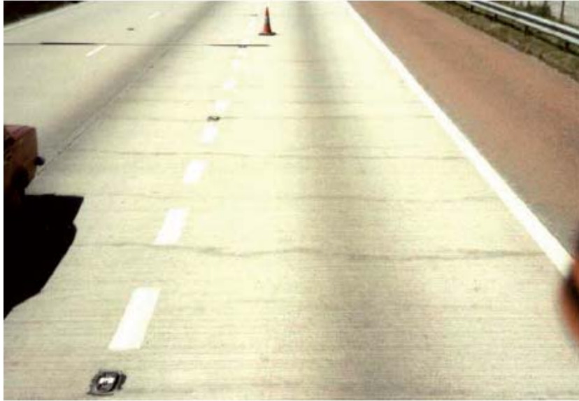
(a) closely spaced tight transverse cracks
