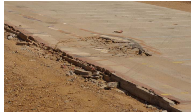
HVS testing typically continues until a failure condition is reached.
