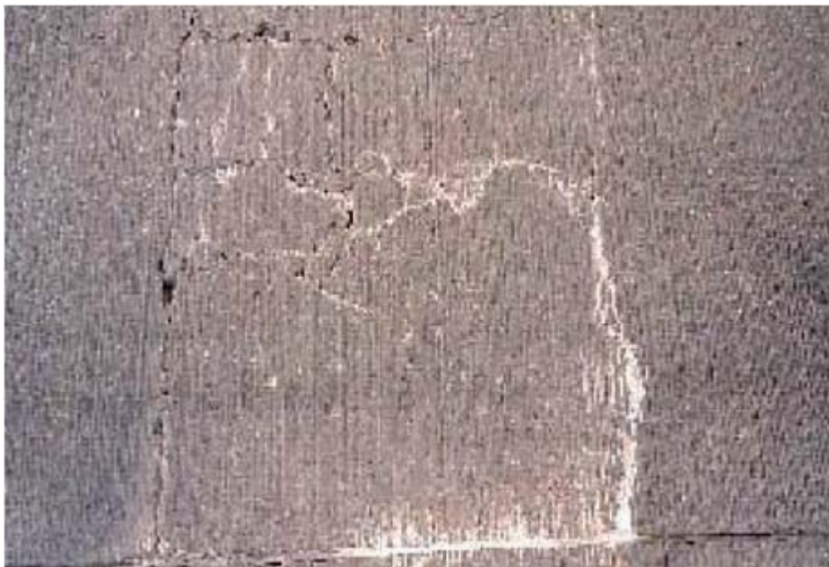
(b) Intersected crack pattern
