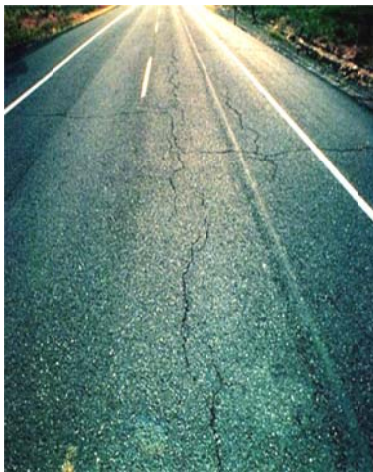
Low Severity (Source: Pavement Interactive)
