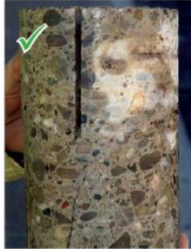
(b) Compliant core: Fine, full-depth, vertical crack
