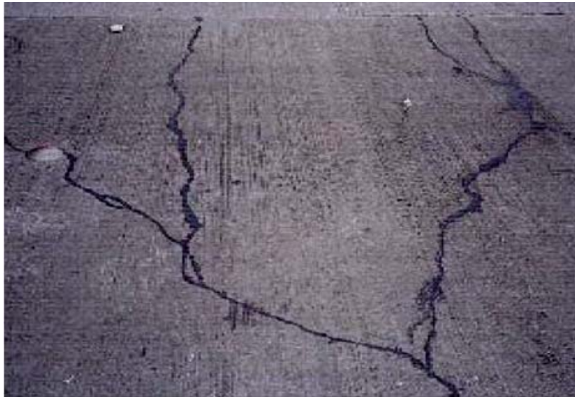
(b) tight bifurcated cracks
