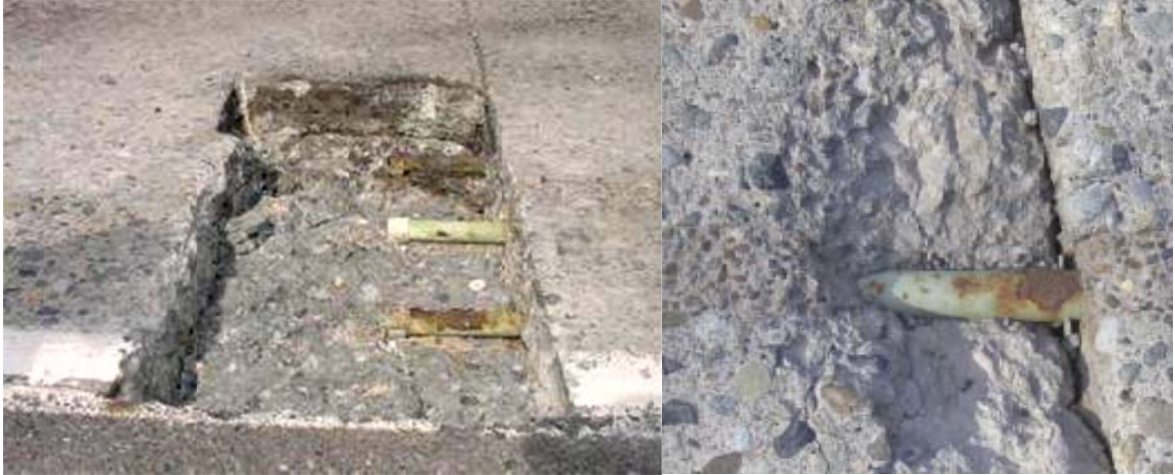
Figure 19. Corroded epoxy coated dowel bars in a retrofitted dowel bar project (original bars 1.5" by 18"). (Photos: WSDOT)
