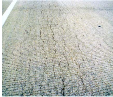
Advanced Stage of Cracking (Source: N. Jackson)
