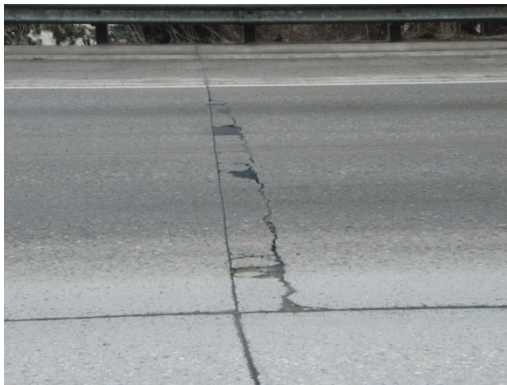
Failed contraction joint due to dowel misalignment
