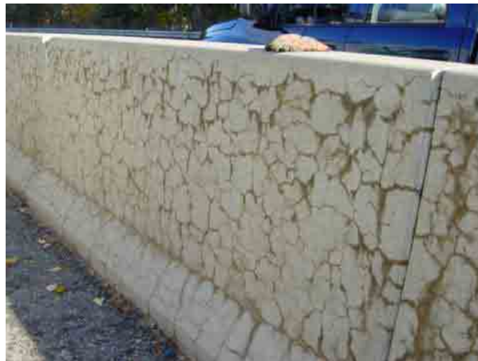
Figure 17. Illustration of ASR on a traffic barrier. (FHWA)
