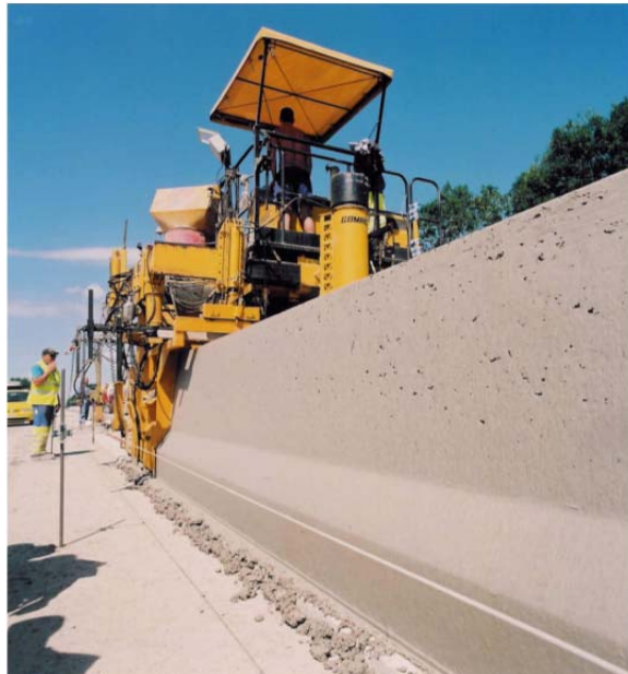
Figure A.24. Slipform paving of the safety barriers on the E40/A10 CRC overlay project. (Photo: Hall 2007)
