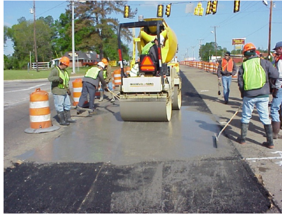
Figure 6. Construction of RMP. Application of the grout to the open-graded HMA. (from Battey and Whittington, 2007)
