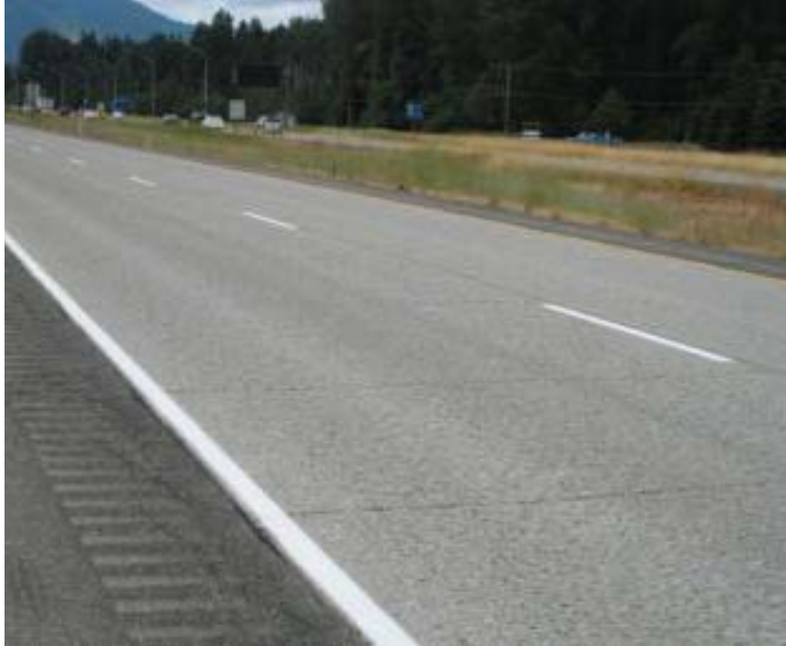
Figure 22. Unbonded 9 in. JPCP concrete overlay placed over concrete (Interstate 90 in Washington State [overlay 35 years old]). (Photo: WSDOT)
