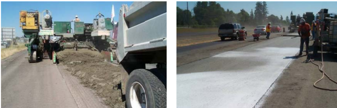
Construction of bonded PCC overlays in July 2003 which were placed directly on rotomilled HMA.
