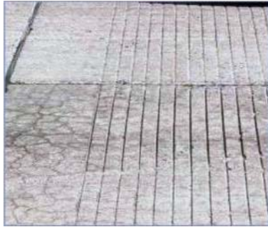
Early State of Cracking (Source: N. Jackson)
