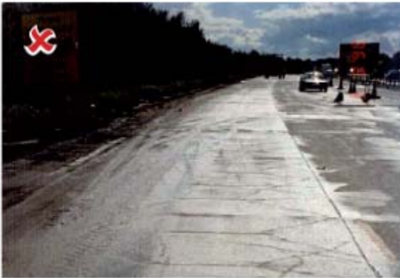
(a) Example showing excessive longitudinal cracking
