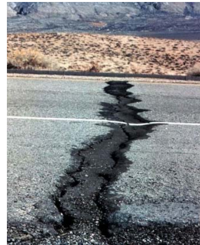
High Severity (Source: Pavement Interactive)
