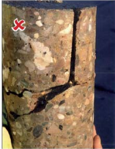
(a) Non-compliant core: Steel reinforcement not severed
