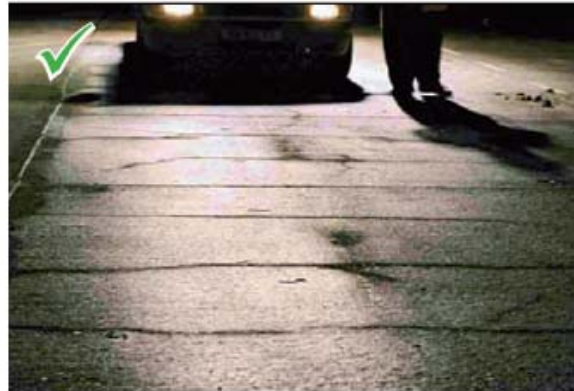
(b) Example showing good transverse cracking
