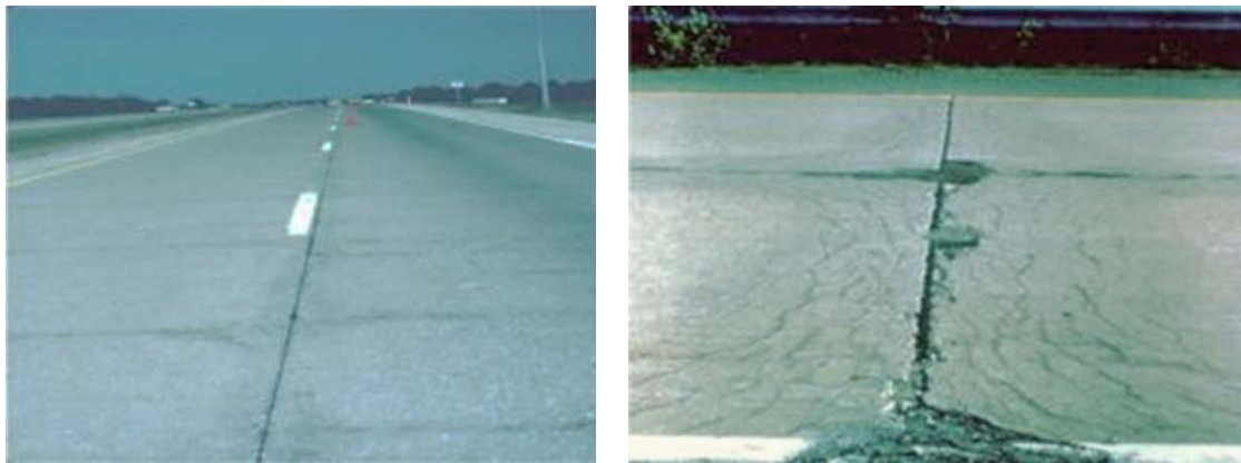
Figure 15. Photos illustrating D-cracking. (Sources: FHWA, NHI)
