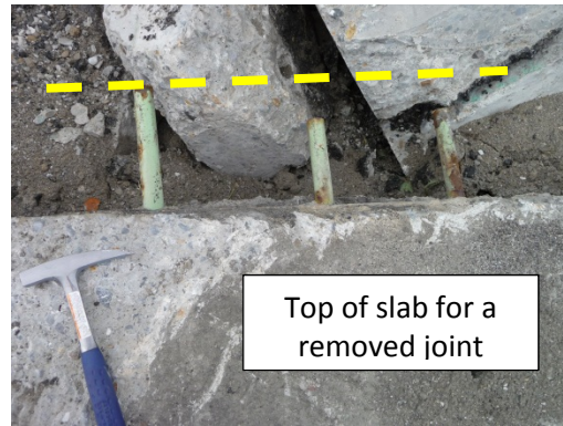
Example of dowel longitudinal translation (joint is not the same as the one to the left)
