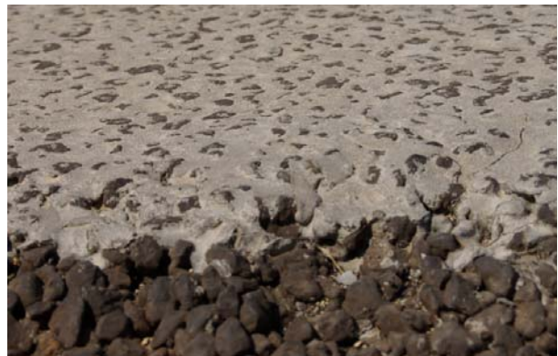
A close-up of the resin modified cement which was placed on open-graded HMA.
