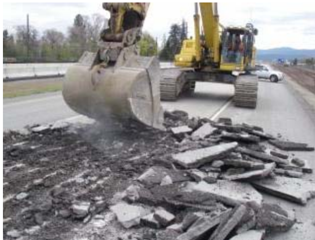
Removal of 3 in. PCC overlay prior to reconstruction of this portion of I-90
