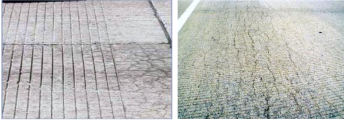
Figure 18. Illustration of ASR in concrete pavements. (Source: D. Huft, South Dakota DOT)
