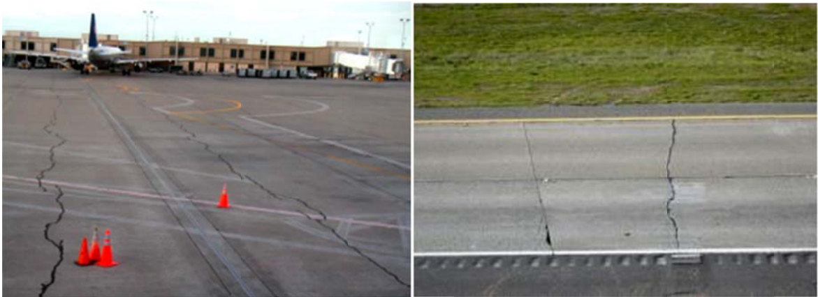
Figure 26. Illustrations of transverse cracking on an airport apron and an Interstate Highway. (Photos: Joe Mahoney)
