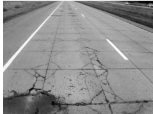
MnRoad Cell 94. Bonded concrete overlay 3 in. thick with a 4 ft by 4 ft joint spacing in November 2003.
