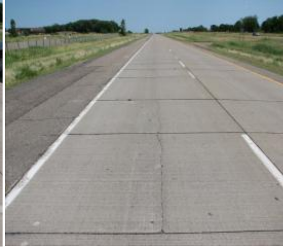
MnRoad Cell 97. Bonded concrete overlay 6 in. thick with a 10 ft by 12 ft joint spacing without dowels. Performance: excessive faulting and some longitudinal panel cracks resulted in replacement of this section in 2010.
