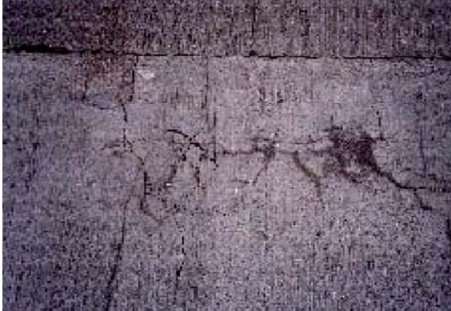
(a) Spalled cracks
