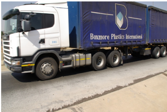
Resin modified pavement at a truck weigh station on the N-3 near is near Johannesburg, South Africa.
