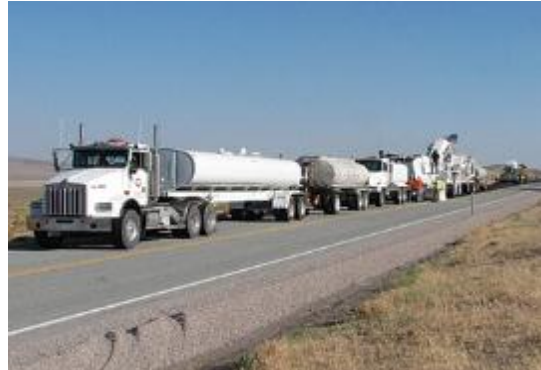
(b) CIPR Train with addition of lime slurry or cement in slurry
