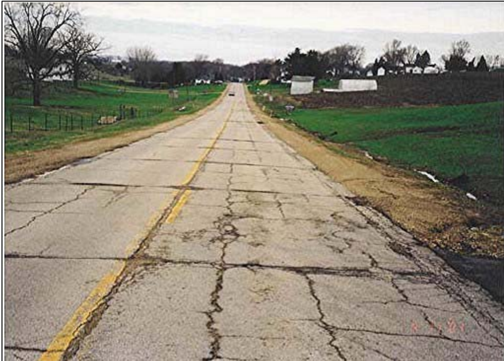
Figure A.15. Reflection cracking in HMA overlay over PCC pavement (Martin, 1973).
