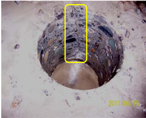
(e) Compliant crack illustrated by core hole
