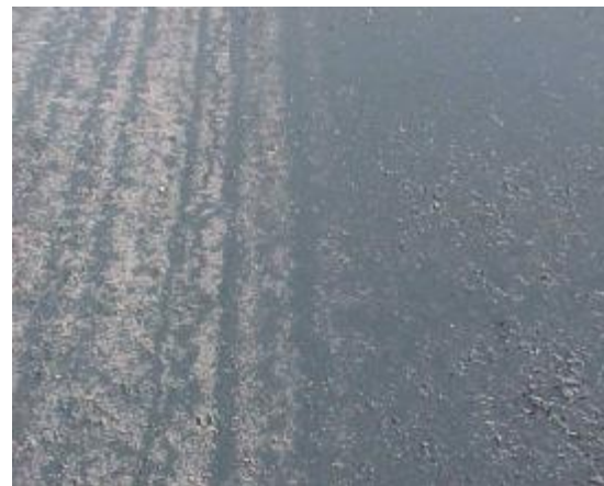
(b) Poor tack coat (left portion of photo)
