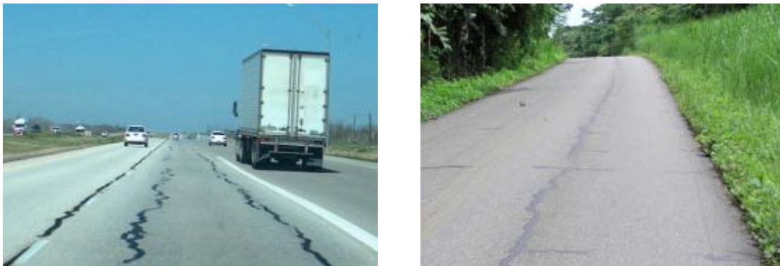
Figure 29. Illustration of longitudinal top-down cracking following crack sealing for a US Interstate Highway (left) and longitudinal and transverse top-down cracking in Panama (right).
