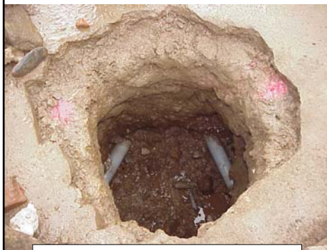
3 conduits interfere with 36" pole footing diameter
