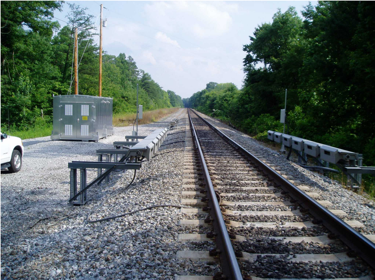
Figure 2: Norfolk Southern test site for wayside detectors in Flat Rock, Kentucky
