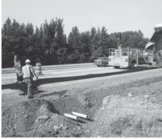
Drainage pipes installed along edge of the Interstate collect and remove water that soaks into pavement layers; renewed attention to underdrain materials, design, and inspection is preventing problems caused by temperature fluctuations.
