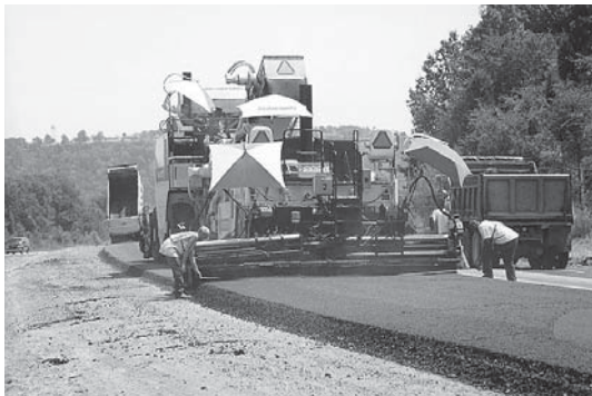
Arkansas road work crews use stringline to double-check thickness, grade, and slope of the laydown of coarse first layer—or base course—of ACHM. Each successive layer uses more finely crushed aggregate.
