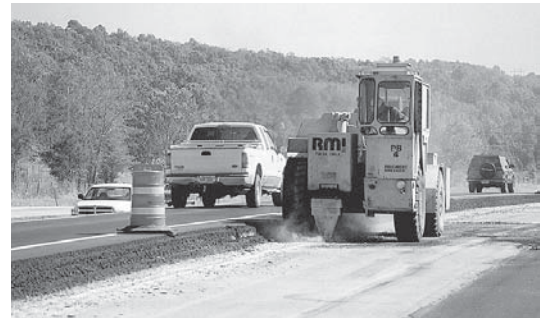
Rubblizing allows reuse of deteriorating pavement: resonant breaker head reduces old concrete surface to rubble, which is compressed with vibratory roller and becomes the bed for layers of asphaltic concrete hot mix (ACHM).
