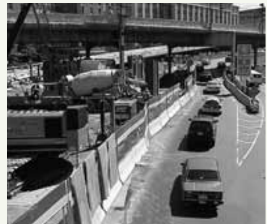
Reconstruction of urban roadways—above, near Boston, Massachusetts—is often difficult, dangerous, and expensive.
