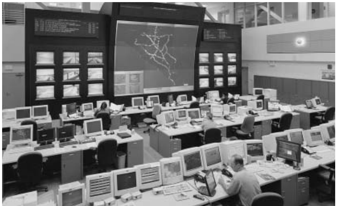
Transportation management centers regulate travel on streets and freeways and maximize levels of service.
