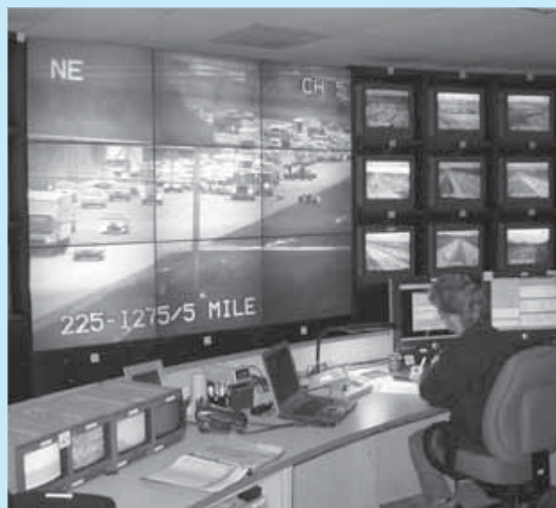
A contract operator works in the control room at the Michigan Intelligent Transportation Systems Center.
