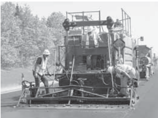
Microsurfacing is one of many pavement preservation techniques that states are integrating into a plan of preventive maintenance, rehabilitation, and reconstruction.
