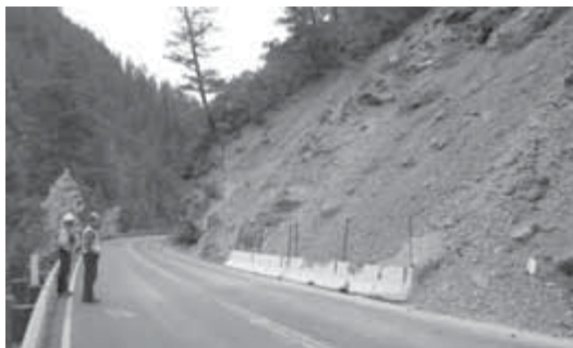
Caltrans engineers perform a slide stabilization project on US-199 near the Oregon border.
