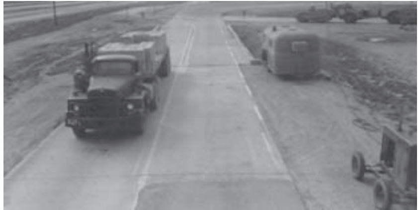
Loaded truck crosses test bridge. Bridge trailer that housed data recorders is at right.
