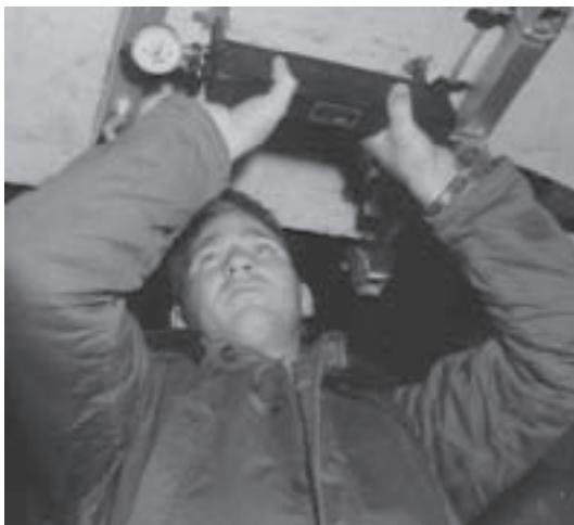
Installing sensor beneath a bridge. Sensors were connected to data recording equipment in trailer.
