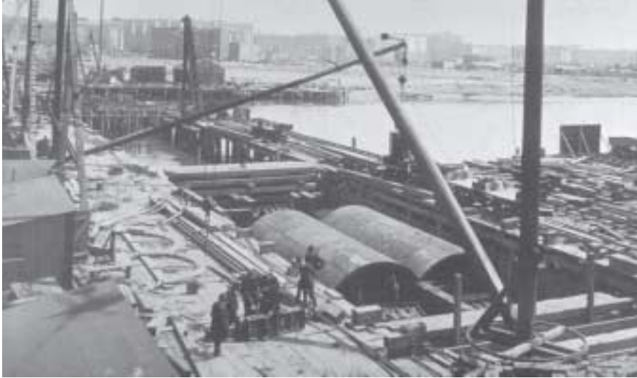
Construction of the tunnel under the Harlem River to connect Manhattan and the Bronx used an early version of the immersed tube method.
