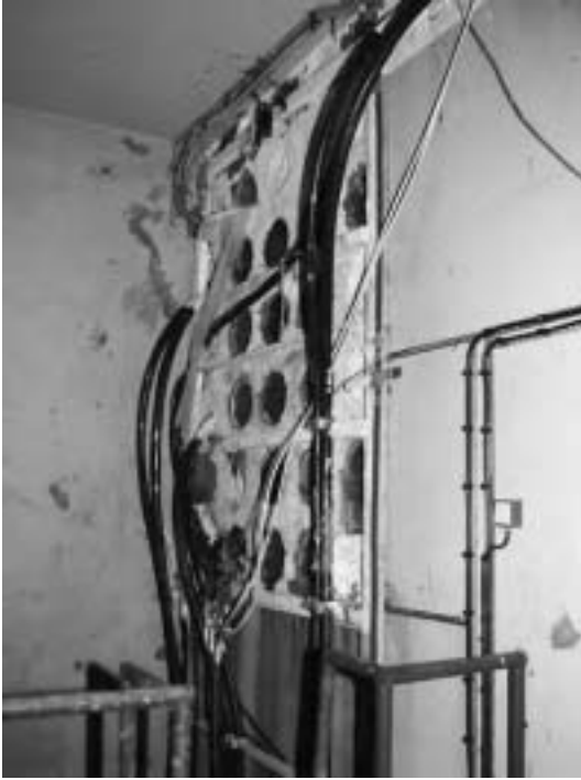
Broken cable seals were evident after the 2002 floodwaters were pumped from the stations.
