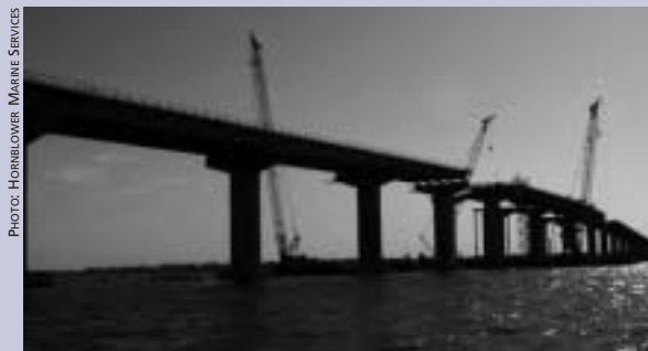
Remnants of the I-90 bridge (left) in Bay St. Louis, Mississippi, after Hurricane Katrina in August 2005, and the new bridge nearing completion in spring 2007.
