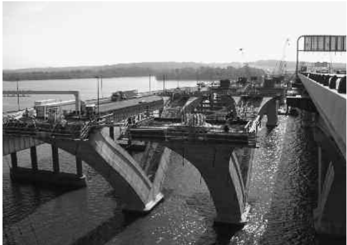
Construction of the new Woodrow Wilson Bridge on I-95 and I-495 across the Potomac River near Washington, D.C., proceeded as traffic continued on the old bridge ( left ) and on the completed span ( right ).
