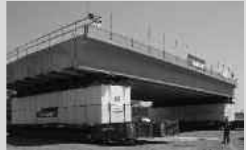
Graves Avenue span over I-4, northeast of Orlando, Florida, was installed in minutes with self-propelled modular transporters.
