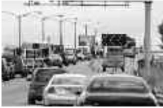
Minimizing traffic disruptions and maintaining work zone safety during necessary bridge repairs calls for innovative strategies.
