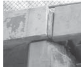
Bridge damage from magnitude 5.4 Chino Hills earthquake.
