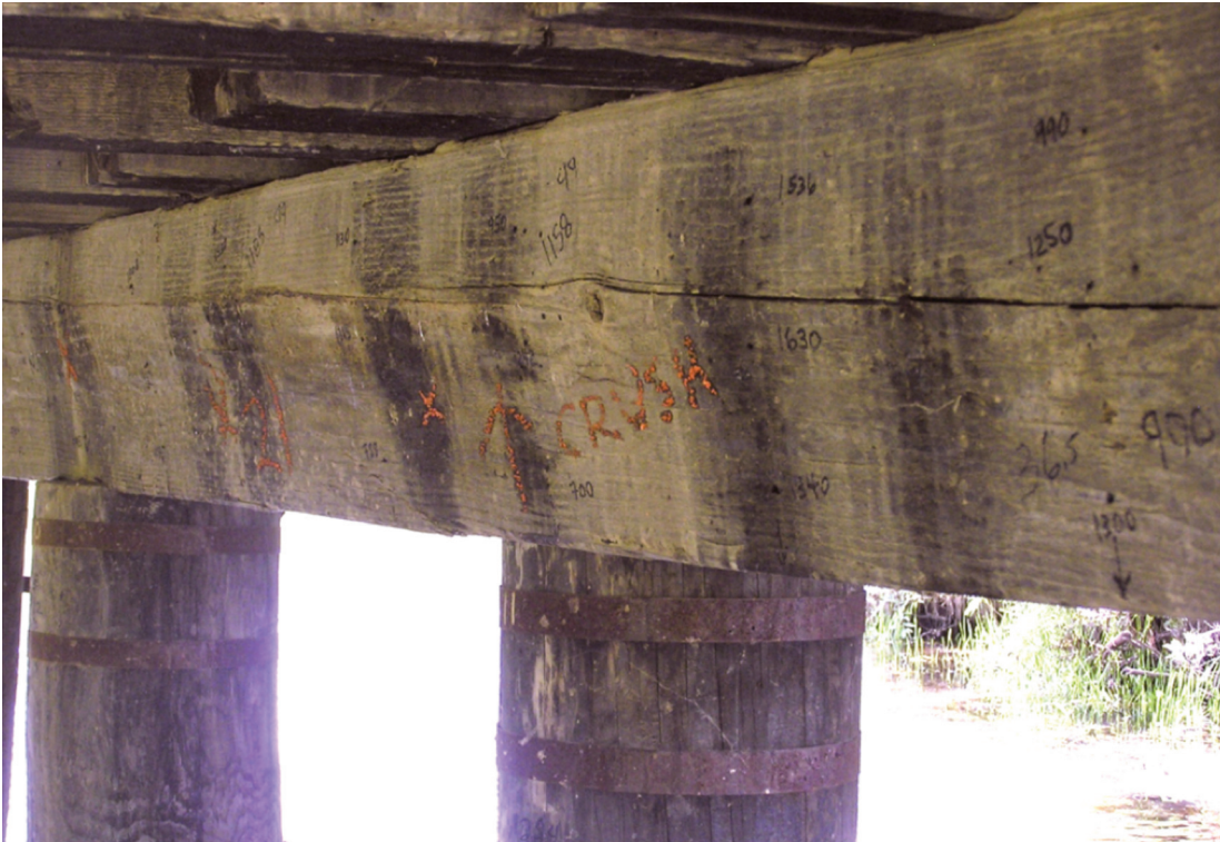
A long horizontal split provides an opportunity for moisture to pass through the timber deck and enter the abutment cap, leading to substantial decay.
