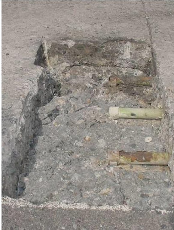
Epoxy coating quality
