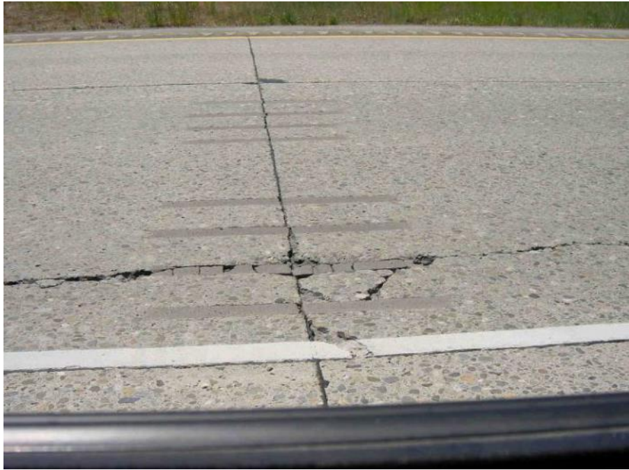
Longitudinal crack intersects dowel bar slot
