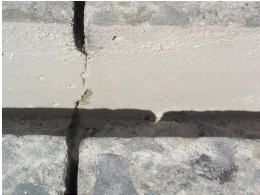
Prior to cleaning
